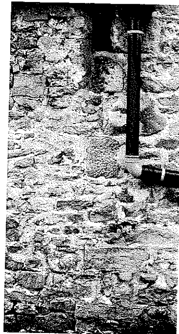
Quoins to be reinstated at the junction with the shippon
