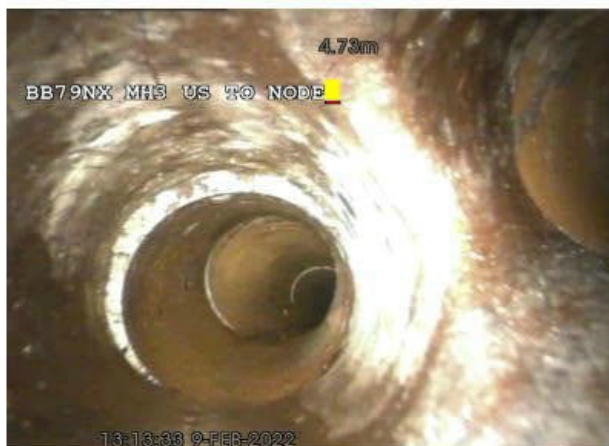
8-1-3A, 00:00:21, 4.73 m Large displaced joint
