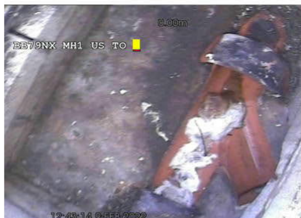
1-1-1A, 00:00:00, 0.00 m Start manhole, MH1, LARGE DEPOSITS IN MANHOLE INVERT
