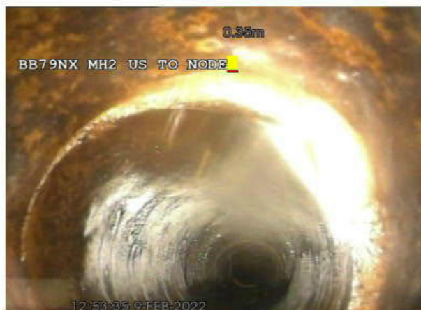
5-1-2A, 00:00:28, 0.35 m Large displaced joint
