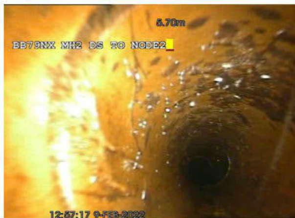
6-1-4A, 00:00:28, 5.70 m Roots at joint
