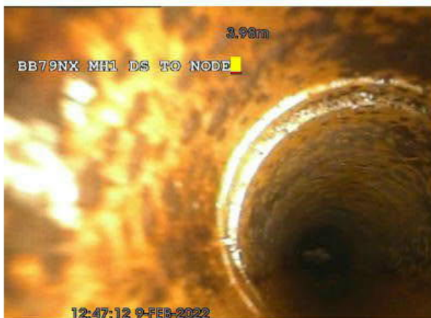
3-1-3A, 00:00:17, 3.98 m Circumferential crack at joint from 6 o'clock to 1 o'clock
