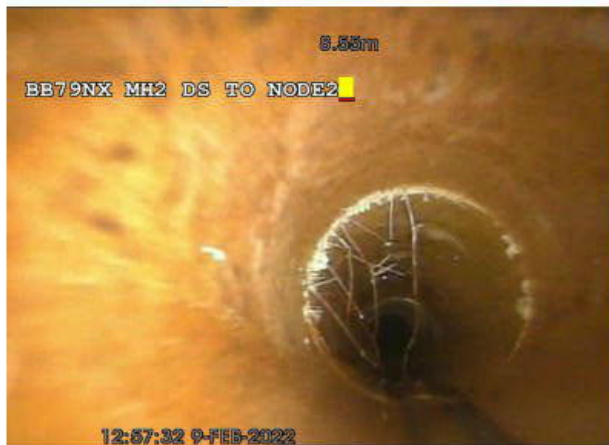
6-1-5A, 00:00:41, 8.55 m Roots at joint
