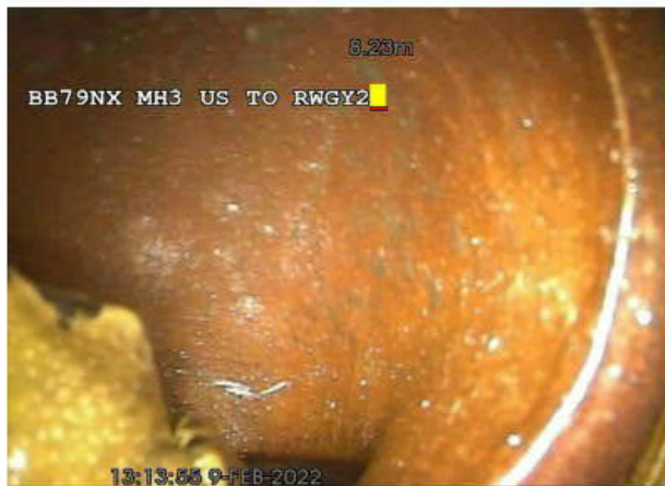
8-1-6A, 00:00:43, 8.23 m Finish gully, GY, the pipe is unserviceable
