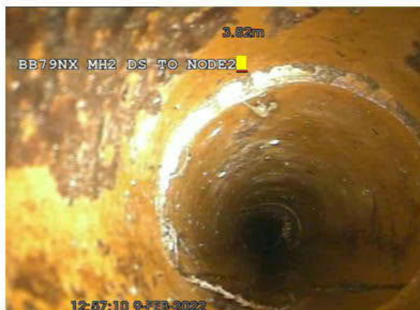
6-1-2A, 00:00:19, 3.62 m Roots at joint
