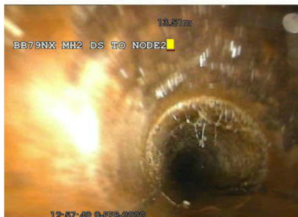
6-1-7A, 00:00:58, 13.51 m Roots at joint
