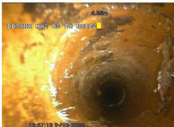
6-1-3A, 00:00:21, 4.35 m Roots at joint
