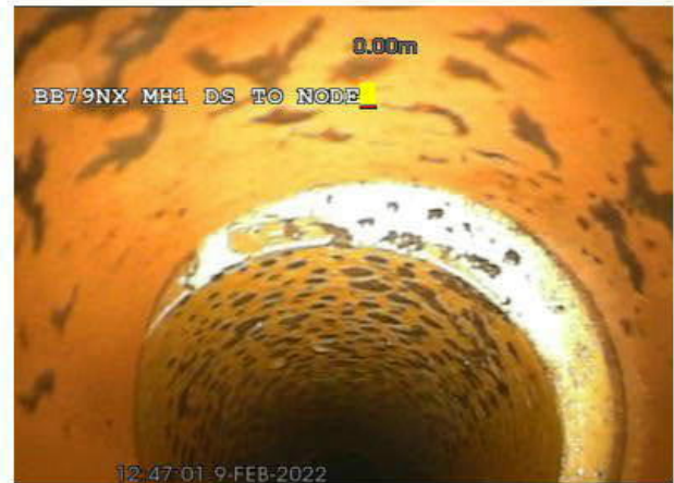
3-1-2A, 00:00:07, 0.10 m Large displaced joint
