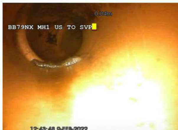
2-1-2A, 00:00:05, 0.04 m Large displaced joint
