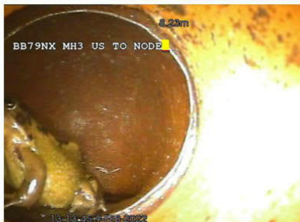
8-1-5A, 00:00:33, 8.23 m General remark, FROG IN PIPELINE
