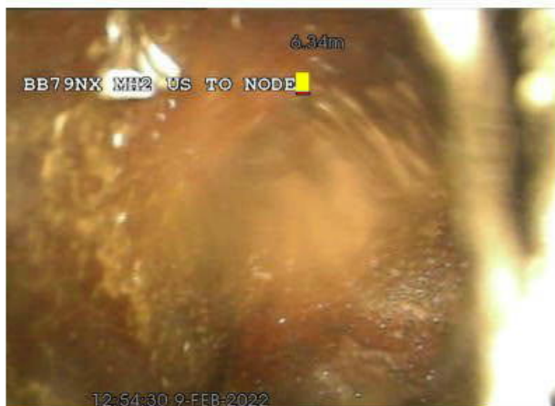
5-1-3A, 00:01:23, 6.34 m Finish gully, UNKNOWN, the pipe is unserviceable
