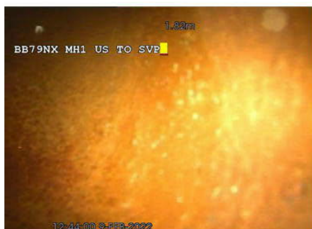
2-1-3A, 00:00:18, 1.82 m Finish gully, SVP, the pipe is unserviceable
