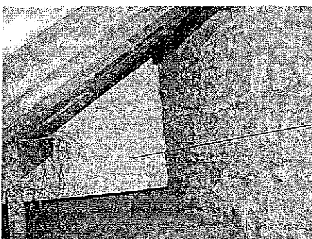
Figure 7: Void D' above the garage
