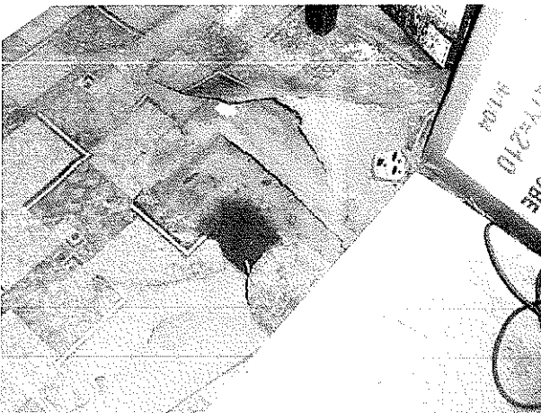
Photograph 29 – Rotten floor proposed to be repaired like for like
