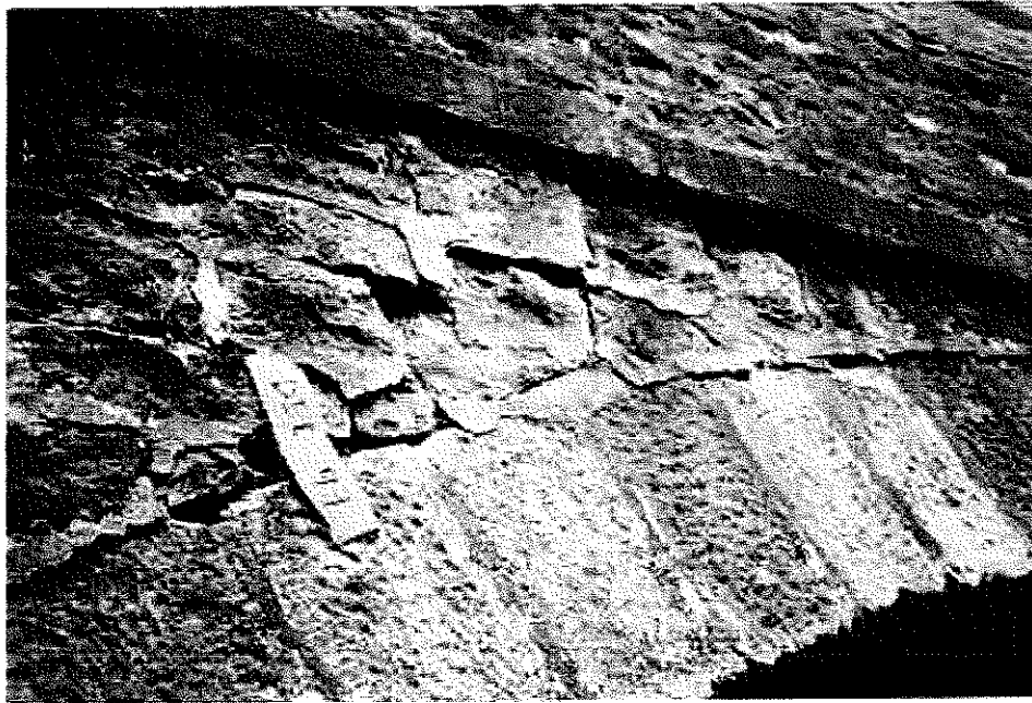
P25 CRACKING/MOVEMENT - WEST ELEVATION OF MAIN ARCH (TELL TAIL NO 1) 29677.3/24
