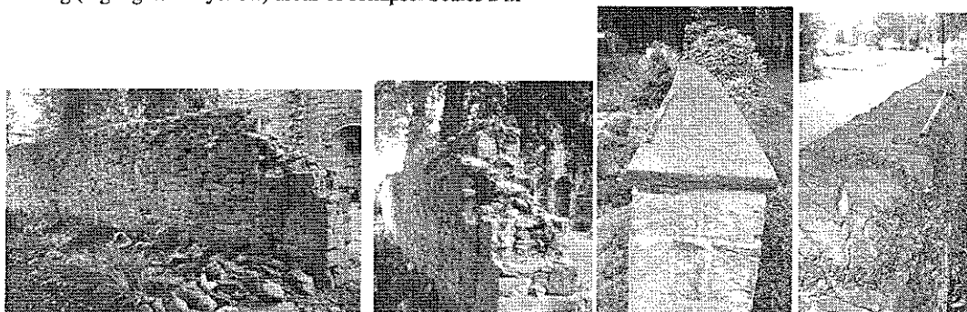
(Left) Fig 17a and b: collapsed S end of east wall; (Centre) Fig 18: recent concrete slab capping of northern part of east wall; (Right) Fig 19 older 'slobbered' concrete wall-head of north wall, parallel to The Sands. Scales 2m
