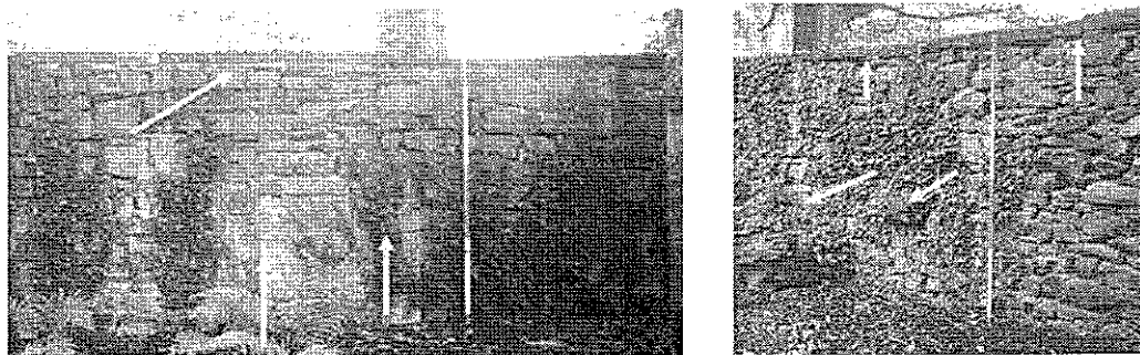
(Left) Fig 23: repaired stretch at east end of south wall, showing pale cement, and blocked doorway; (Right) Fig 24: very large original capping stone, and through/projecting stones, in south wall (Scales 2m, 500 mm divisions)
