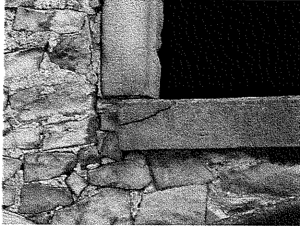
23. Cracking to internal brick wall
