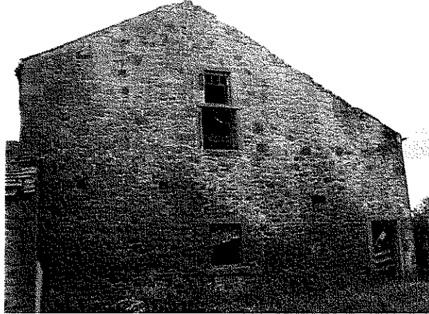
11. Section of northerly gable wall requiring re-pointing
