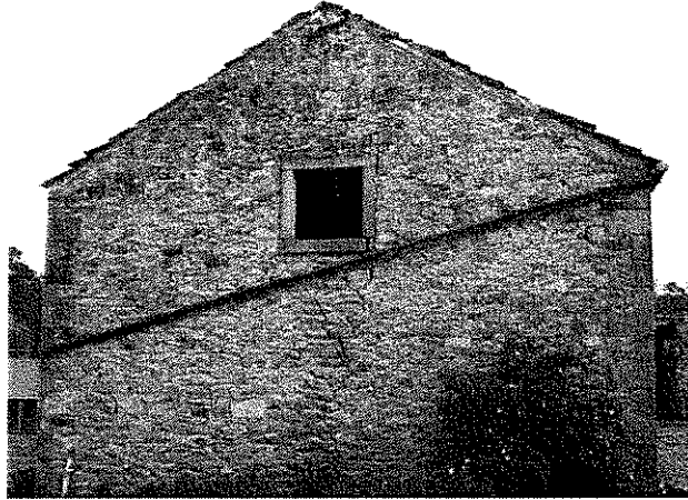
20. Verge detail on southerly gable wall, requiring repair as part of scheme
