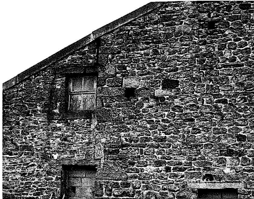
Photo 2 : Signs of differential ground movement / lintel failure
