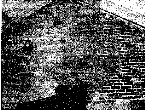
39. Cracking to internal face of external wall to barn 1 noted from within loft area
