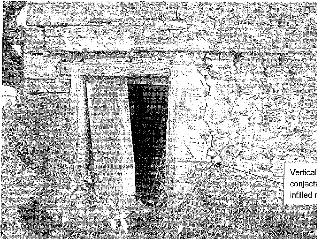
Plate 10. Vertical cracking adjacent to entrance door in Rear Elevation
