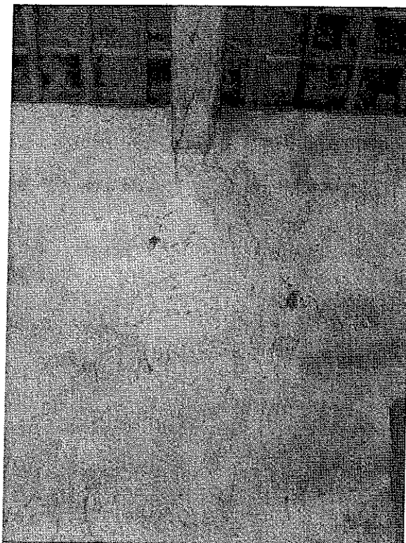
Plate 15. Cracking in render beneath truss bearing
