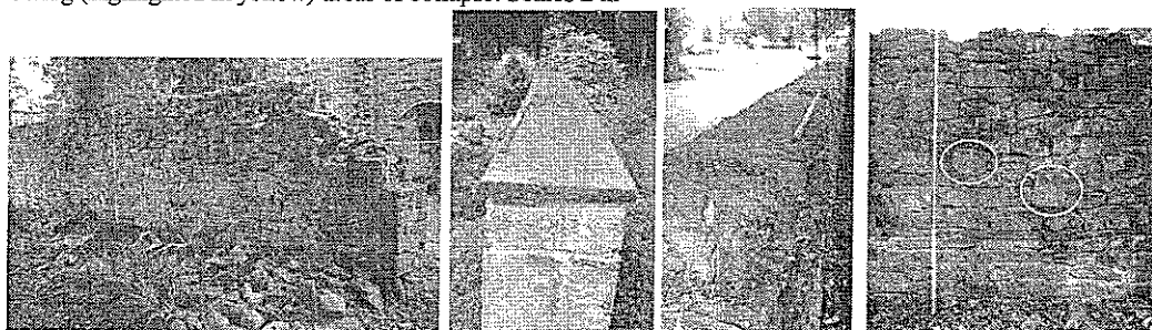
(Left) Fig 9: collapsed S end of east wall; (Centre left) Fig 10: recent concrete capping of northern part of east wall; (Centre right) Fig 11 older 'slobbered' concrete wall-head of north wall; (Right) Fig 12: possible medieval architectural fragments incorporated in the east face of the east boundary wall. Scale 2m, with 500 mm divisions
