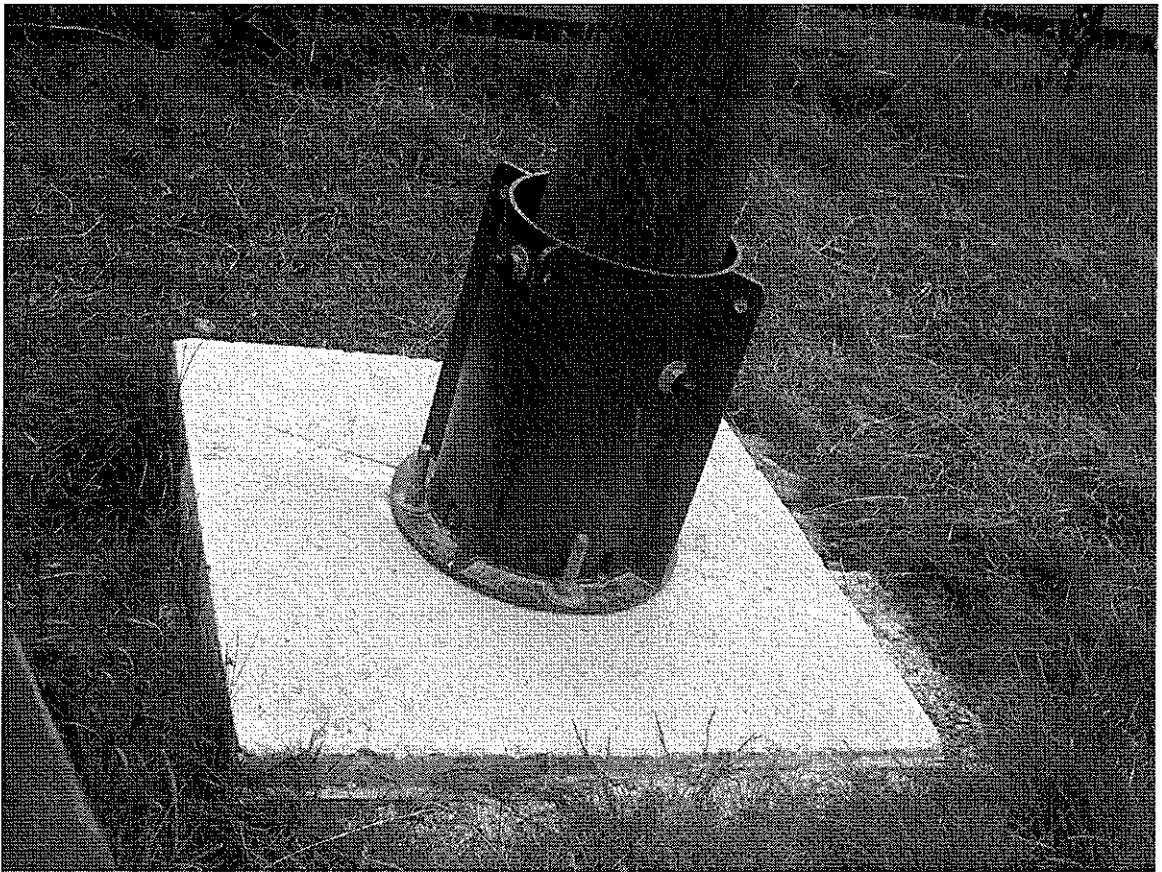
Typical steel shoe for telegraph pole, bolted to concrete base.
