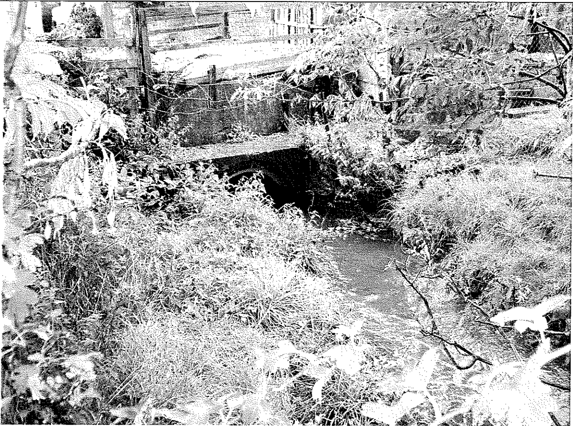
Culvert issues- off site
