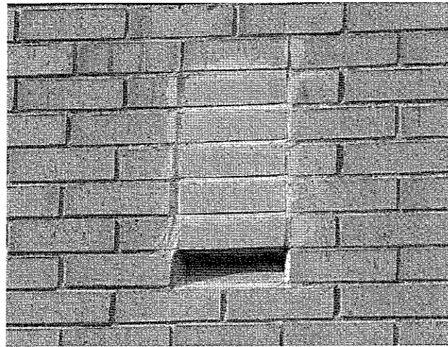
Example of integral wall box to be installed in the Chapel and Sunday School
