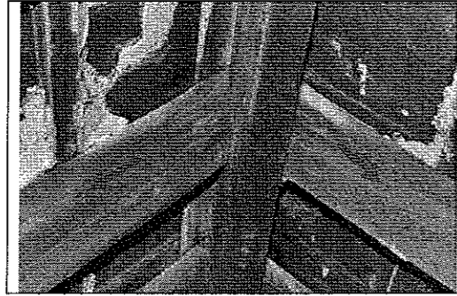
Bat droppings on roof support timbers inside eastern roof void.
