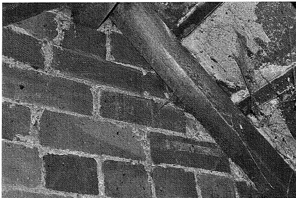
South interior gable – potential roost site and droppings. April 2010
