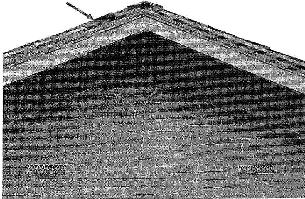
Detail of north gable elevation showing gaps between soffit and wall and gap along top edge of roof. April 2010.
