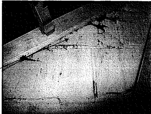
Figure 4: bat droppings on internal wall of roof void
