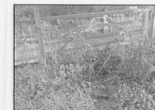
PHOTO 7: Ditch flows under footbridge. Note build up of debris reducing the cross sectional area of culvert.
