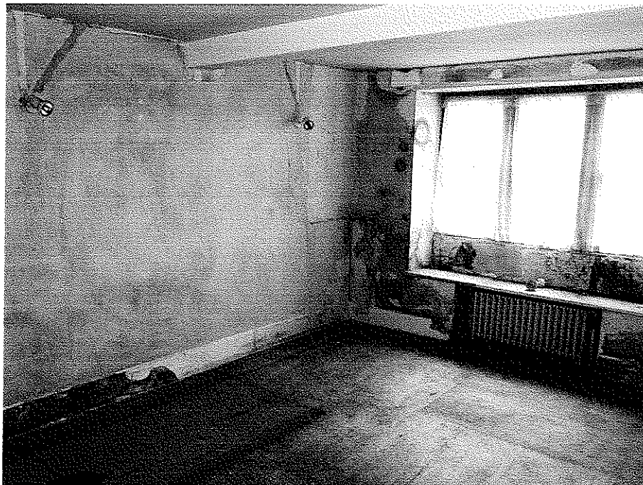
Image 6 - Evidence of serious penetrating dampness and condensation to Dining Room
