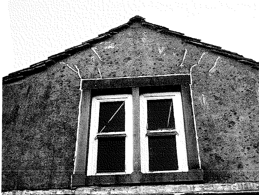
Image 5 - 'sealed' cracking to render, rear elevation
