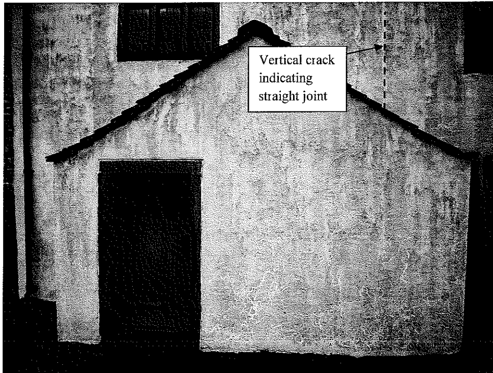
Image 11 - Vertical crack indicating straight joint to front elevation
