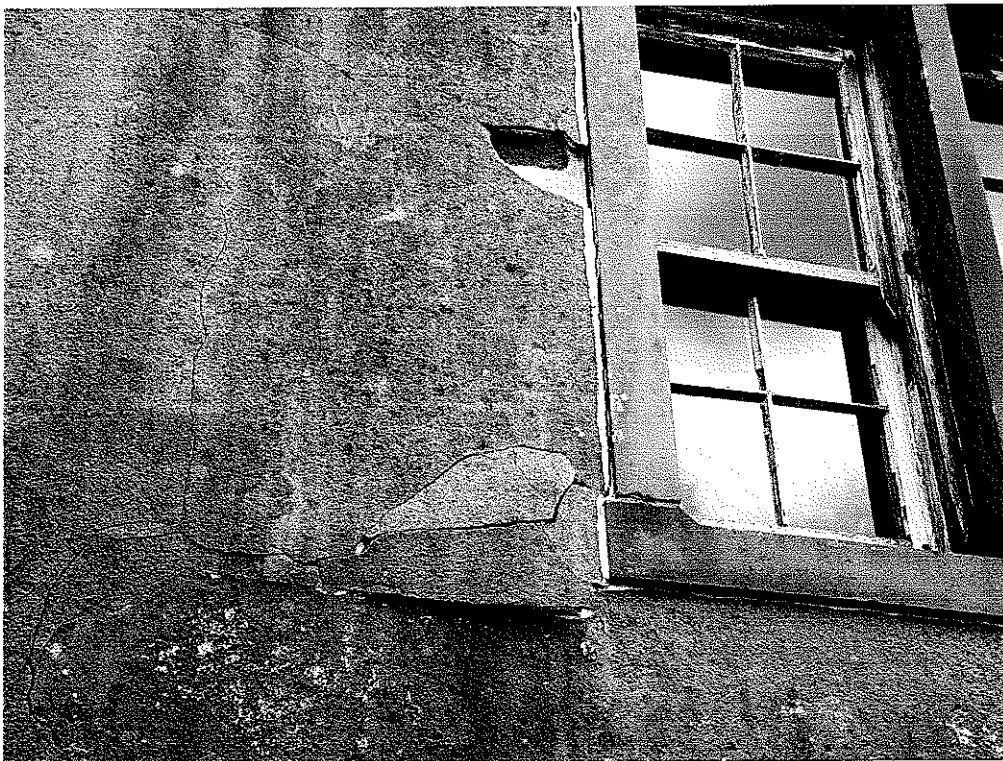
Image 29 – Cracked and detached render to building façade
