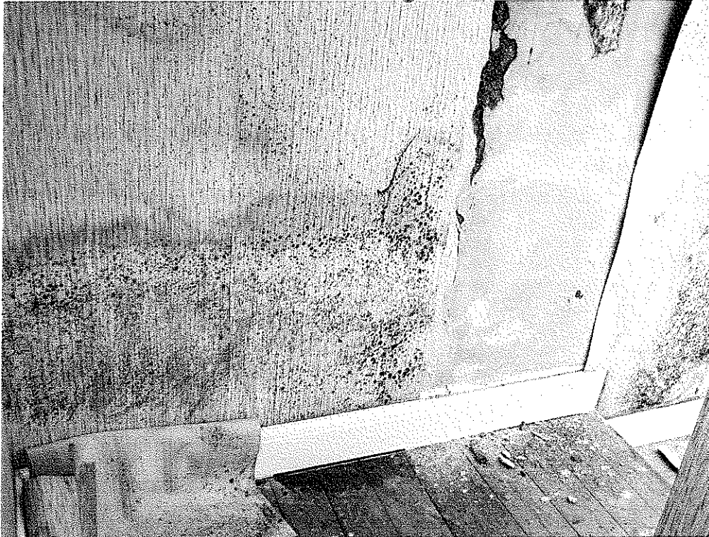
Image 30 – Evidence of serious dampness and condensation at first floor level
