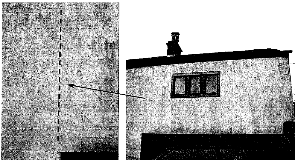
Image 10 - Cracking between original structure and new extension
