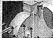
Large Capacity Pumping Stations
