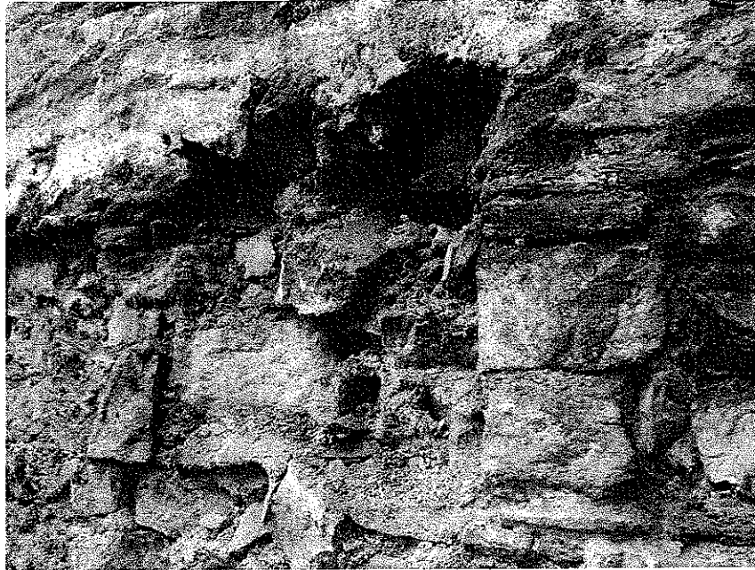
PL 21 Collapsed rubble infill to be re-built
