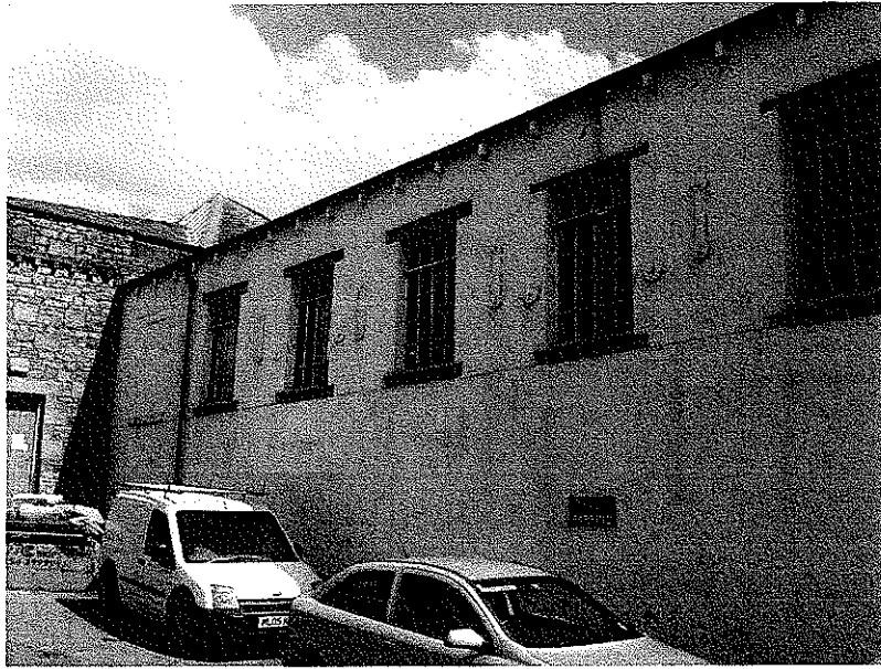
PL. 4 Condition of external wall where rendered
