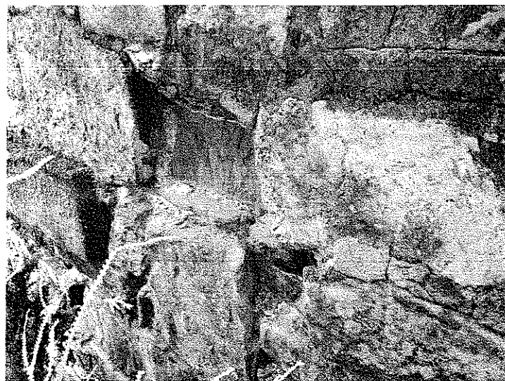
PL. 10 Ledge infill for potential water ingress and weakening of surrounding wall structure
