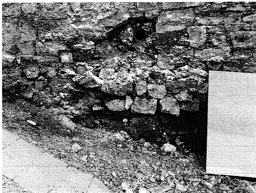
PL 22 Collapsed rubble infill to be re-built due to probibly water ingress due to being below external ground level
