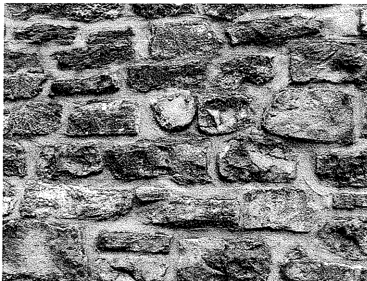
PL. 3 Condition of external wall and pointing generally
