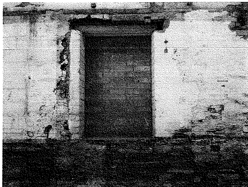
PL 14 Dilapidated structural head and wall surrounds
