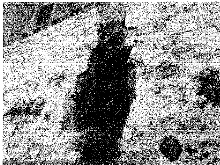
PL 18 Evidence of existing timber floor joist cut off and left in-situ
