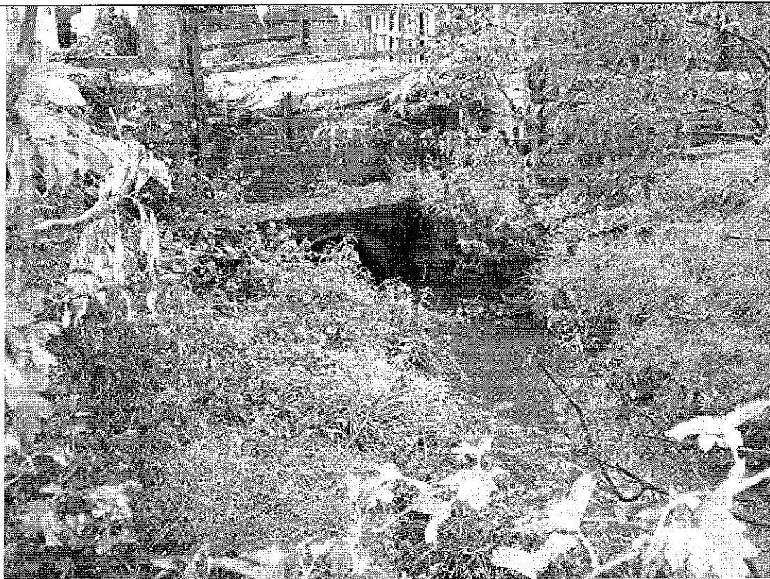
Culvert issues- off site
