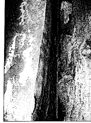
Photo 7.5.3c: Gap at underarch of window lintels
