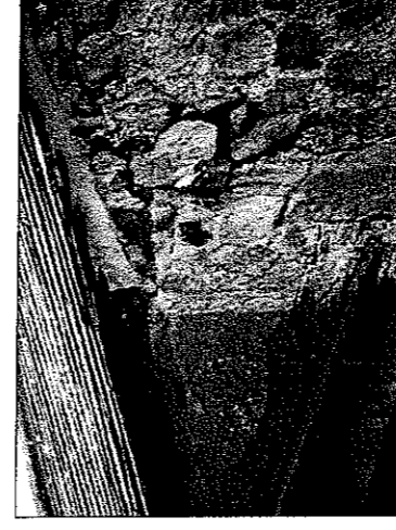
Photo 7.5.2f: Gap in stone work at north-east elevation
