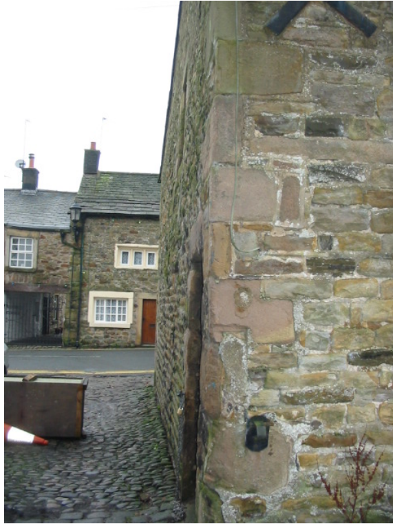
Photo 21 - Distorted Right Gable Wall of Barn
