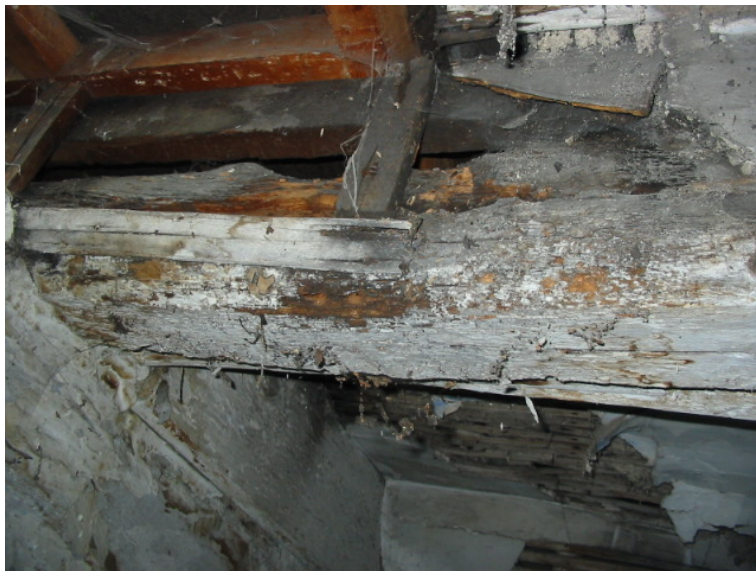
Photo 6 – Decayed Timber Purlin
