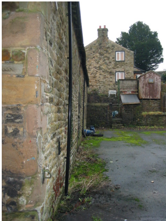
Photo 22 – Distorted Rear Wall of Barn
