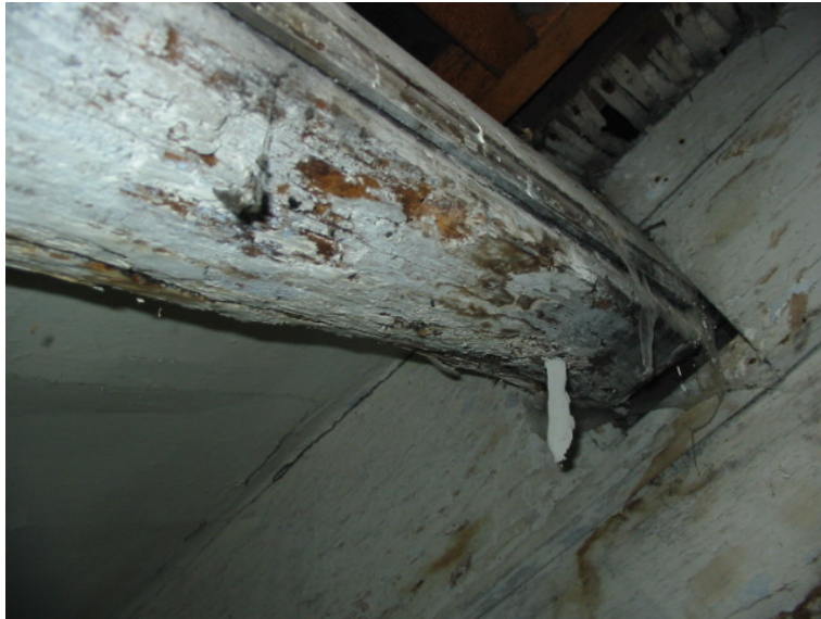
Photo 5 – Decayed Timber Purlin
