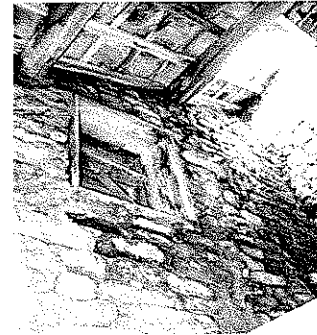
Internal stonework deterioration in barn room to left of main door - note no lintels
