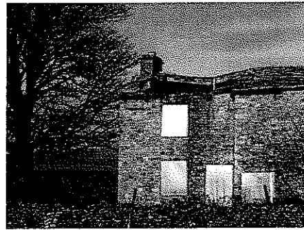
Collapsed roof of later extension to house
