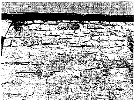
Typical weathering at high level
