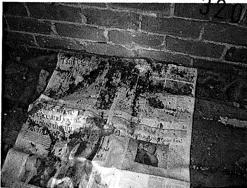
Photo 7 – Photo of droppings on newspaper below ridge at gable end
