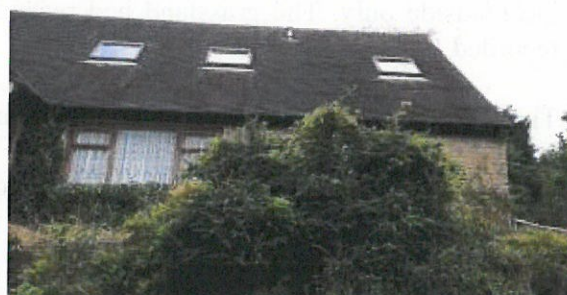
P8: Large section of opportunity to the rear elevation beneath the tiles
