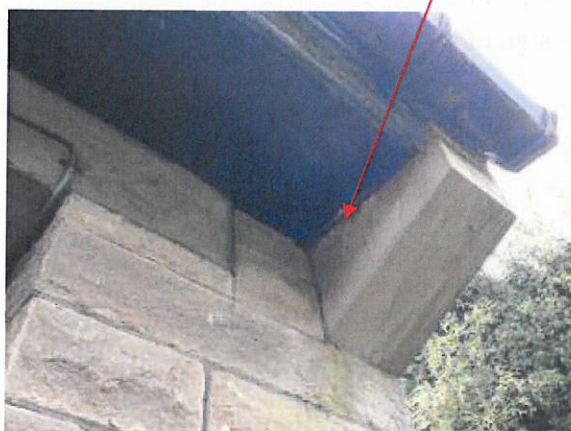
P7: Small gap present between the soffit & stone to the front elevation
