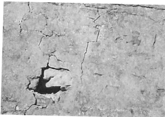
Photograph (1) – Hairline cracks in the render to the south elevation.
