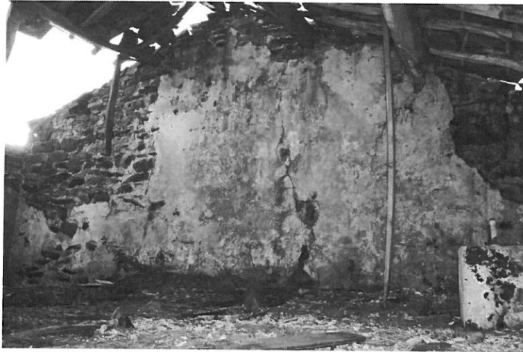
Photograph (17) – Showing plaster missing in the western cottage.
