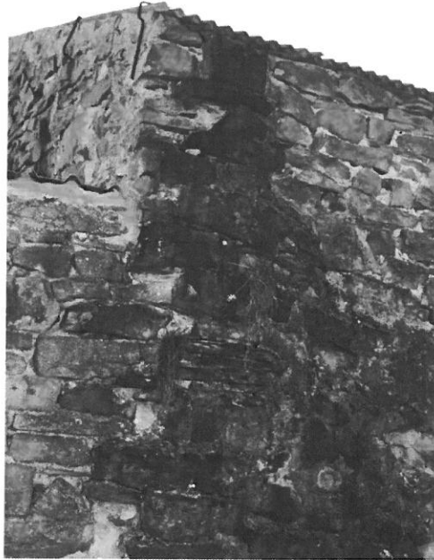
Photograph (11) – North east corner with plants growing in wall.
