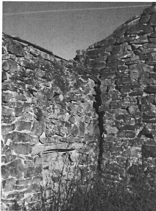
Photograph (13) – Showing the crack at the north west corner.
