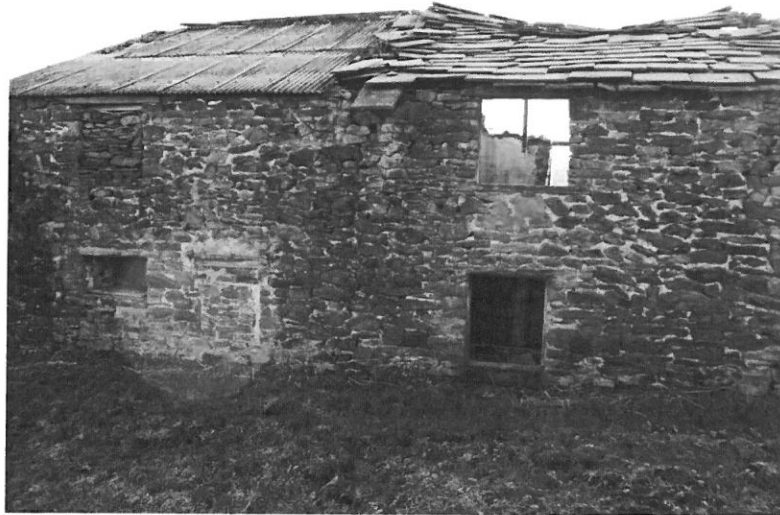
Photograph (8) – North Elevation showing main section of stonework in reasonable condition.
