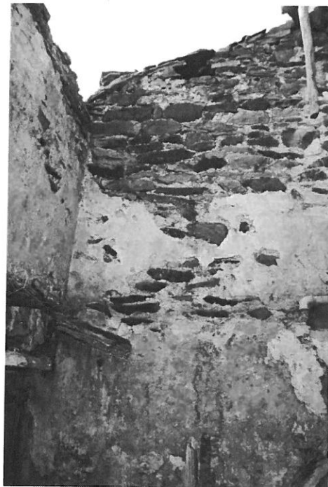
Photograph (16) – Showing some of the collapsed floor to the western cottage and missing plaster.
