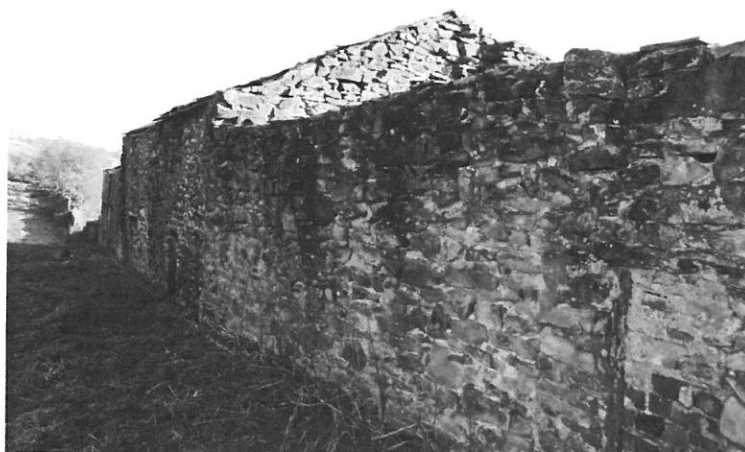
Photograph (12) – Wall forming part of the remains of the fallen down cottage showing the bowing at the top.
