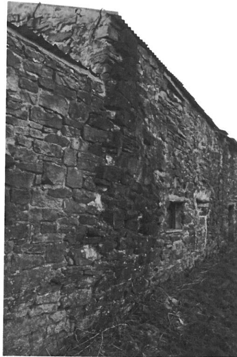
Photograph (9) – North east corner showing slight bow in wall.
