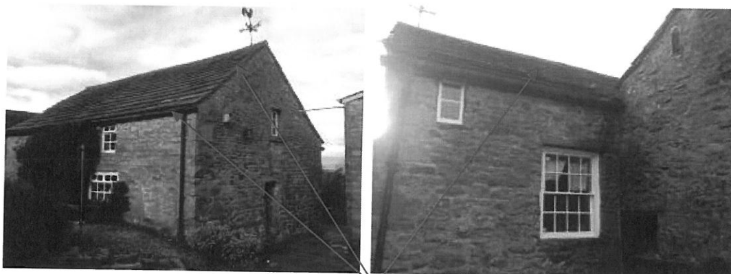
Building 2 – planned to be sold for future development, potential identified between roof tiles, roof verge and fascia board
