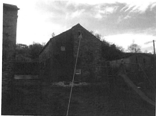
North elevation of building 1 – gap at gable providing access into structure
