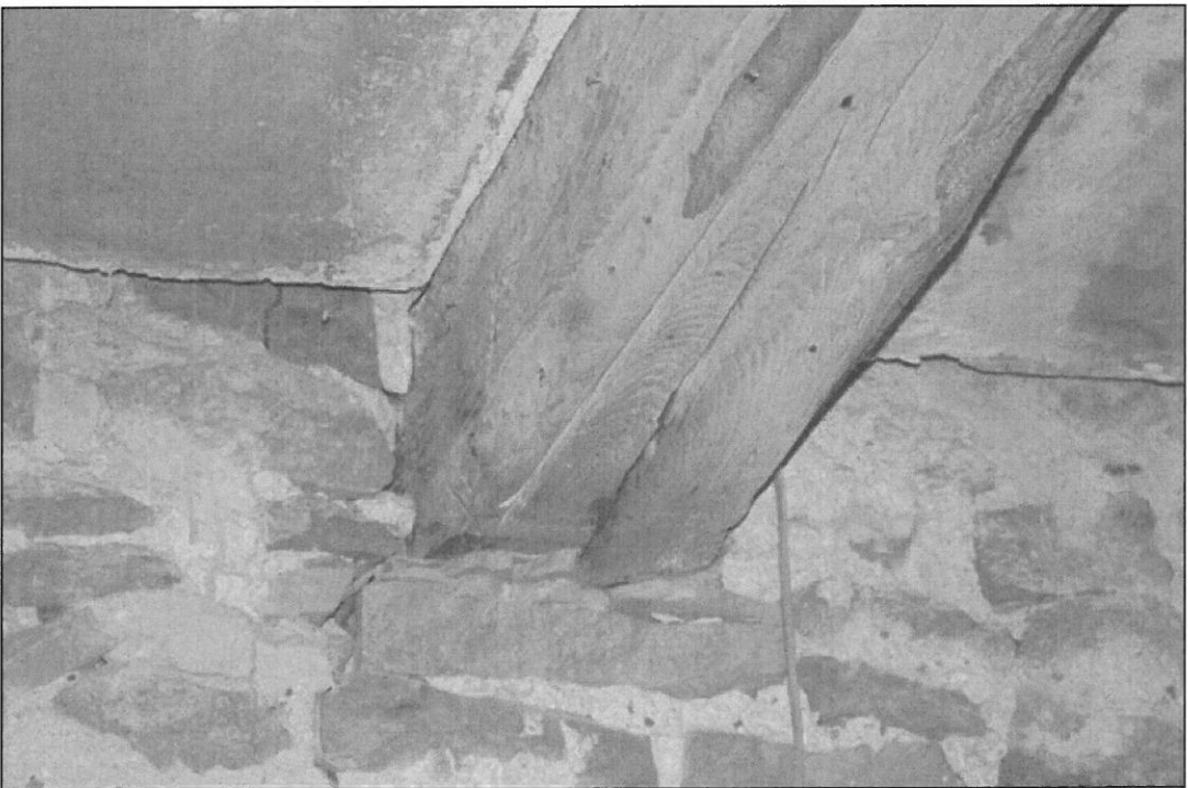
13. Stopped roll- moulded beam on ground floor
