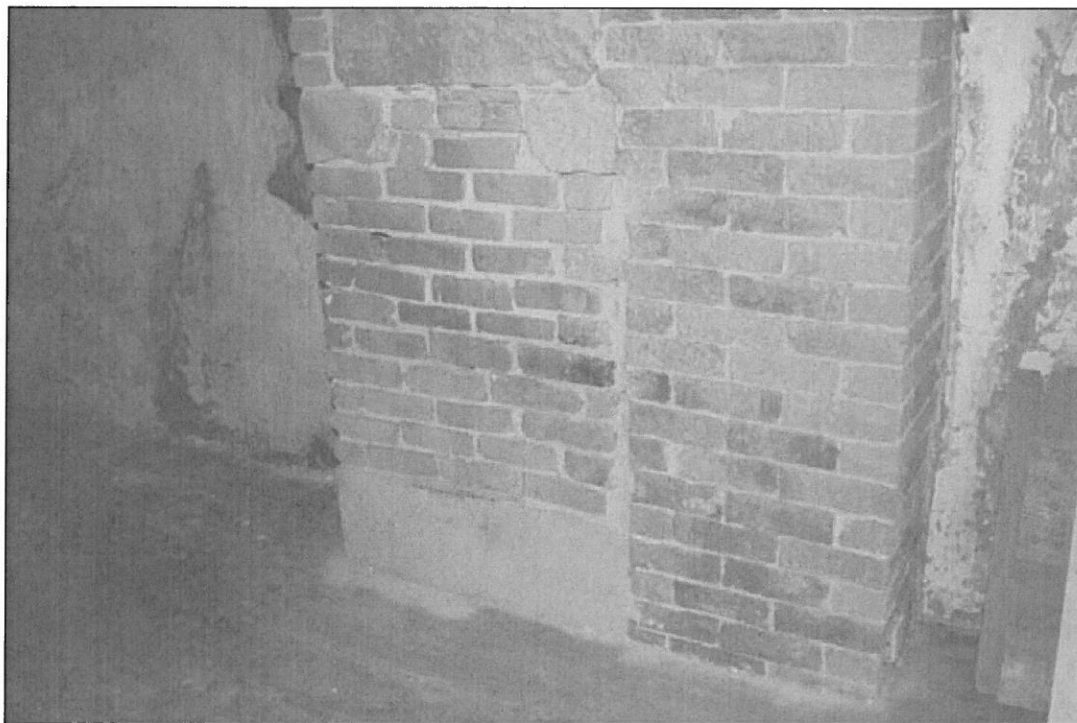
20. Blocked first floor hearth
