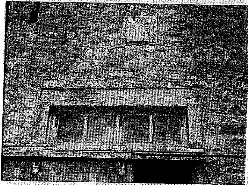
Front Elevation Cracking over Door
