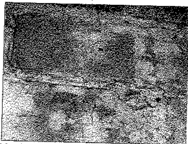
Figure 8 Bat dropping stuck to the wall of the western gable internally.
