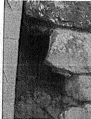
Crevice in stone wall
