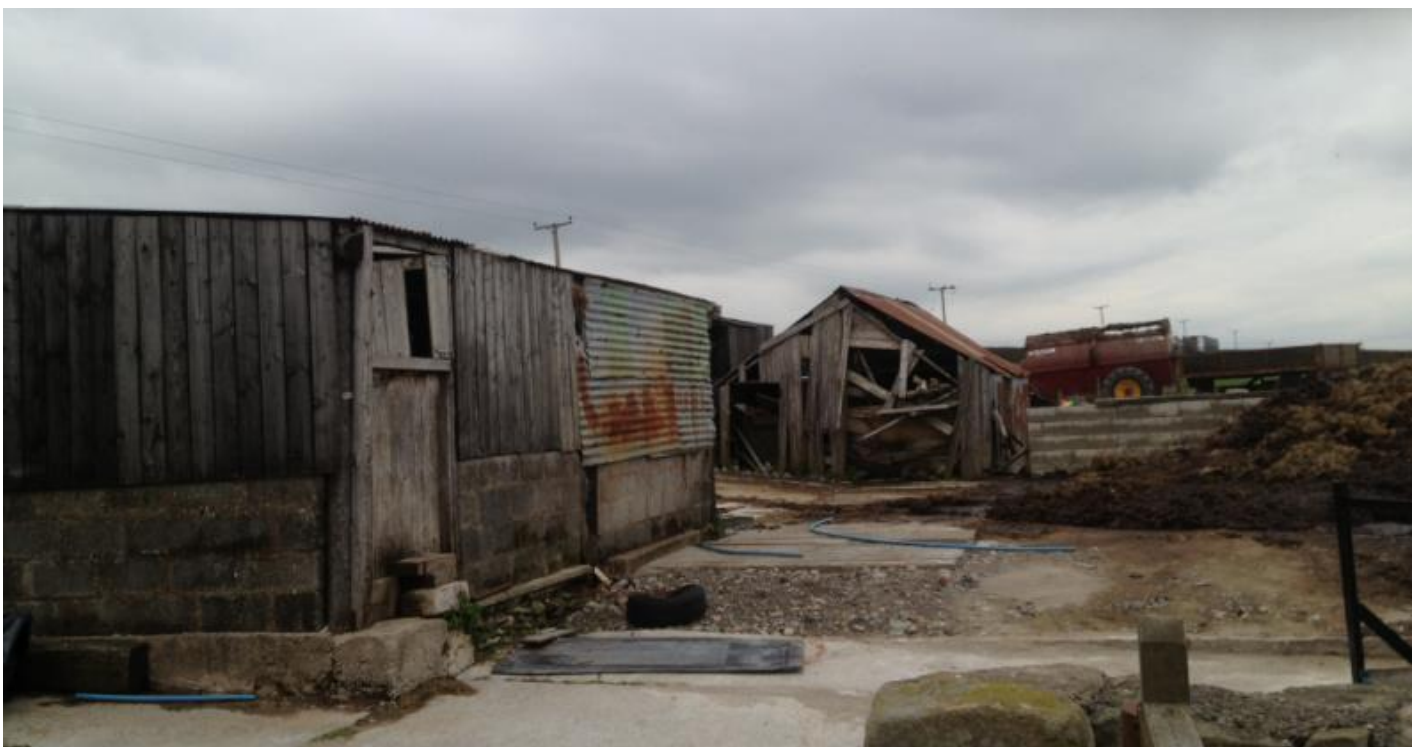
Image of dilapidated sheds and midden.
