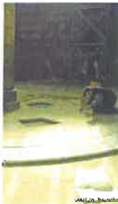
Crack in the floor at Chester Cathedral
