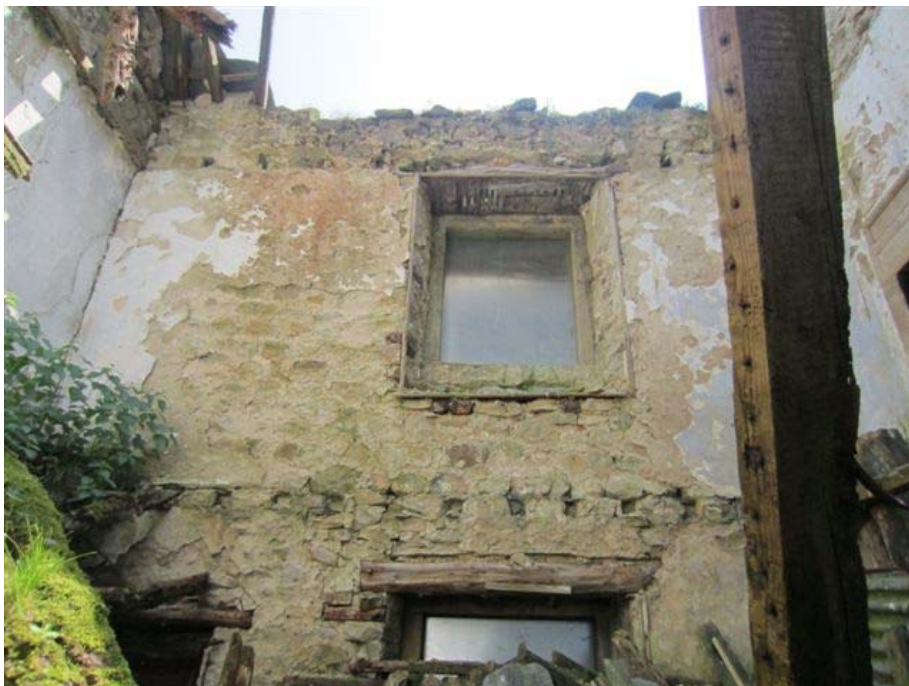
Image 4: Internal view with exposed roof and plaster work in disrepair
