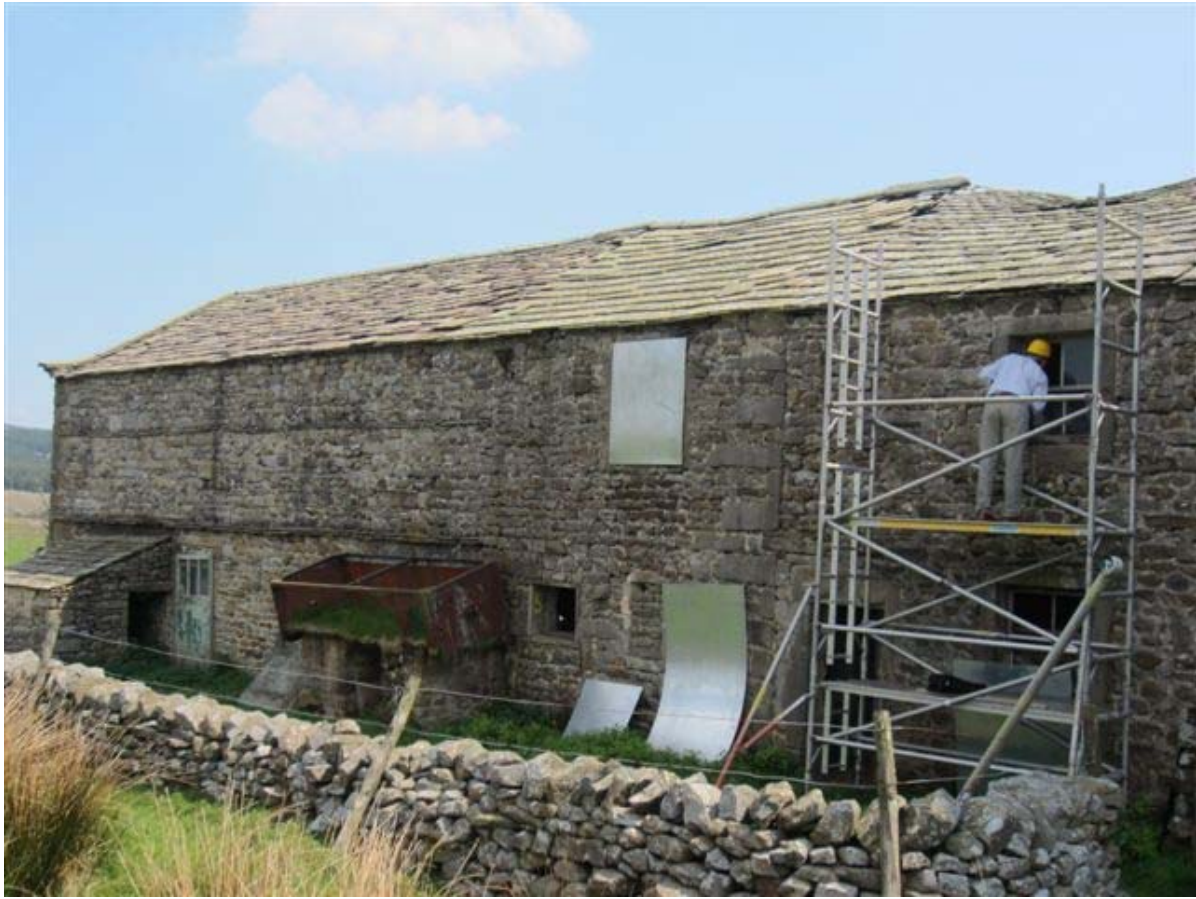
Image 3: Front Elevation view boarded up windows and dilapidated roof
