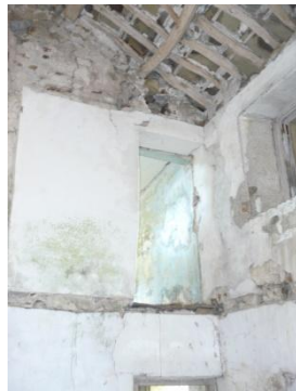
Cracks in wall between houses A and B emanating from the purlin support positions
