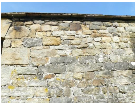
Typical weathering at high level
