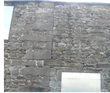
Vertical joint between original house and later extension – noted limited bonding
