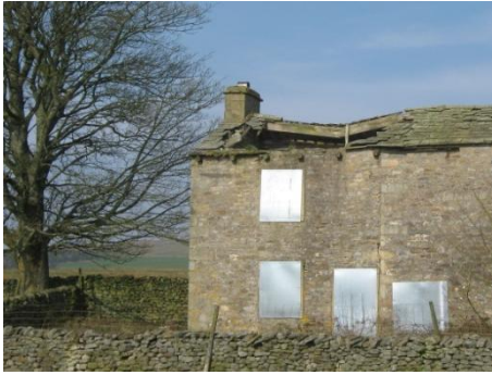
Collapsed roof of later extension to house
