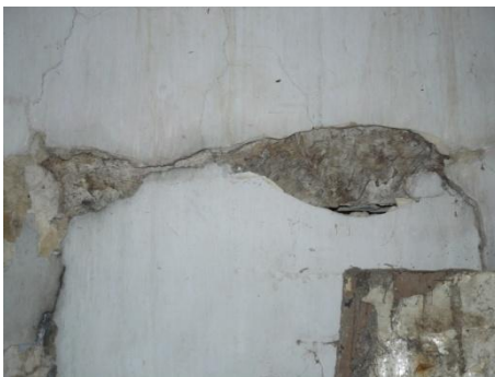
Typical weathering at high level
