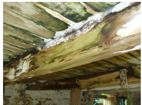
Timber decay in mistal 1 st floor
