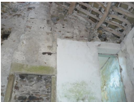
Cracks in wall between houses A and B emanating from the purlin support positions
