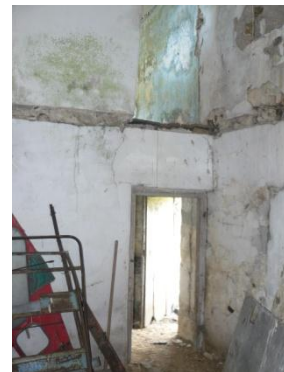
Cracks in wall between houses A and B emanating from the purlin support positions
