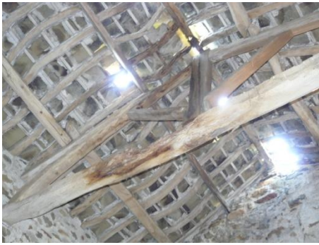
Collapsed roof of later extension to house
