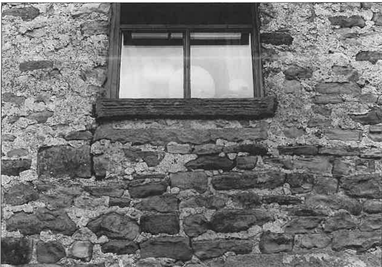
Photo 8: Detail of first floor window sill over housebody, with sill of earlier window below
