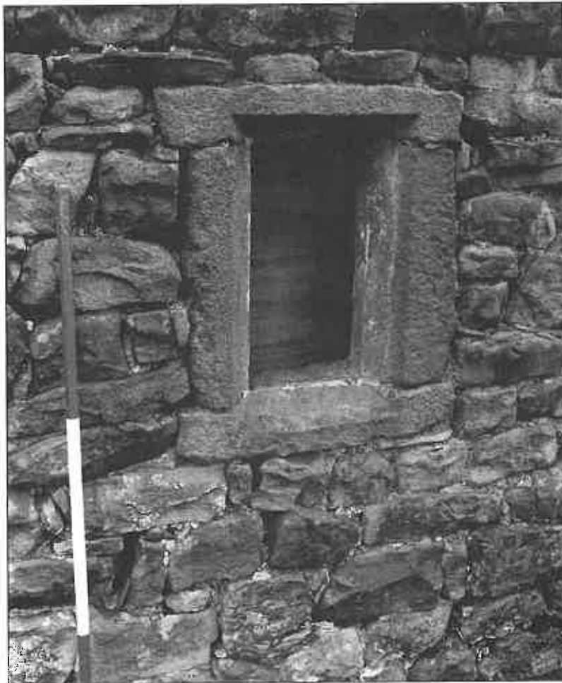
Photo 18: Detail of fire window in north side of housebody
