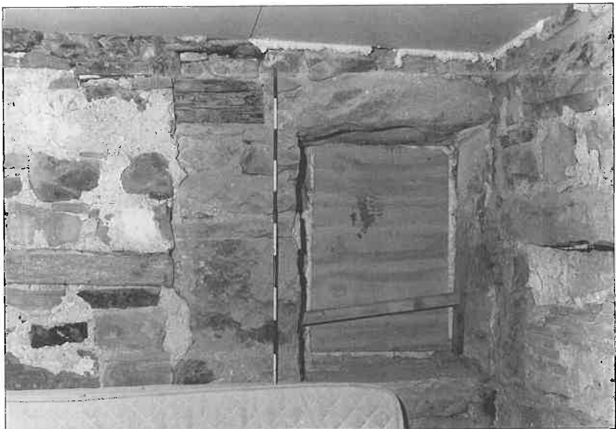
Photo 19: Interior view of fire window and adjacent remains of horizontal timber, in housebody
