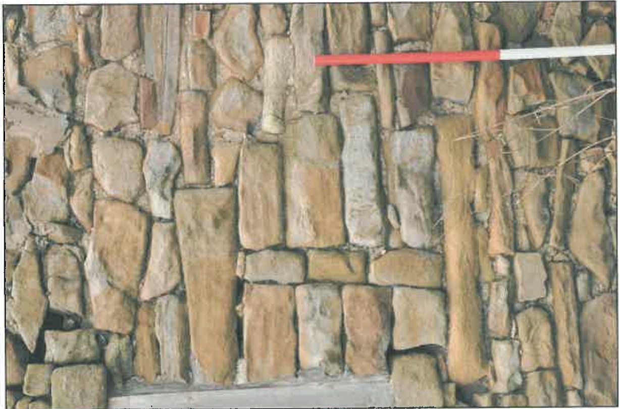
Photo 7: Detail of blocked breather, east side of barn
