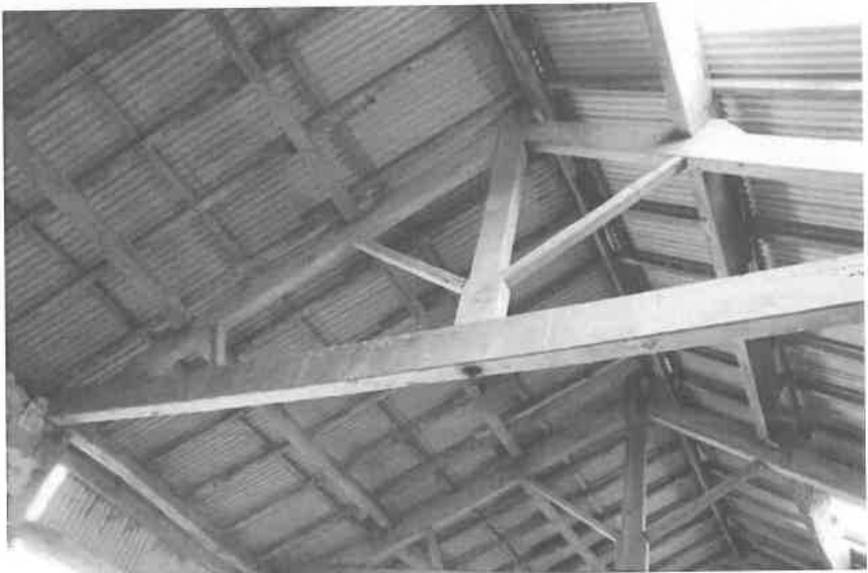
49 The roof structure to the north of the cart entrance, showing the king joggle post and the cleated back purlins.
