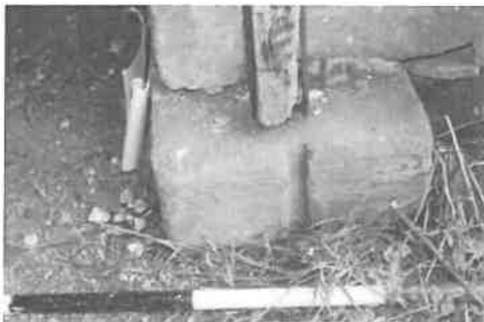
Figure 21 The right hand base of the cart entrance, with the slot for a plank.
