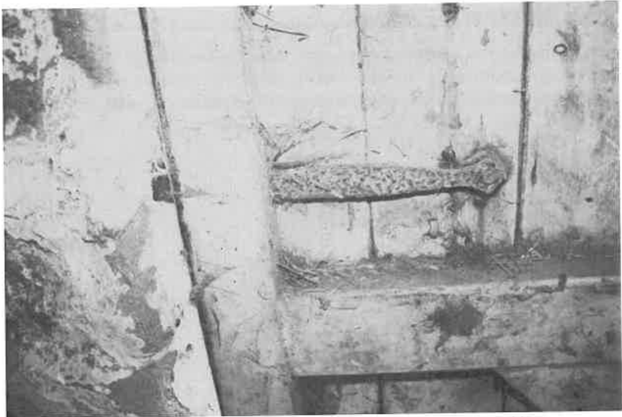
76 An example of one of the metal catches to the doors to the south east gable.
