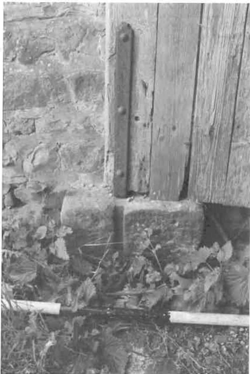
37 The base quoin, with plank slot, to the southern jamb of the cart entrance.
