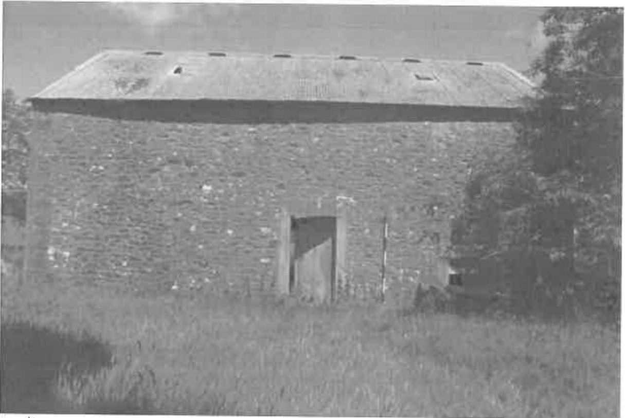
18 The south west elevation, showing the corrugated asbestos cement roof and the door opening.
