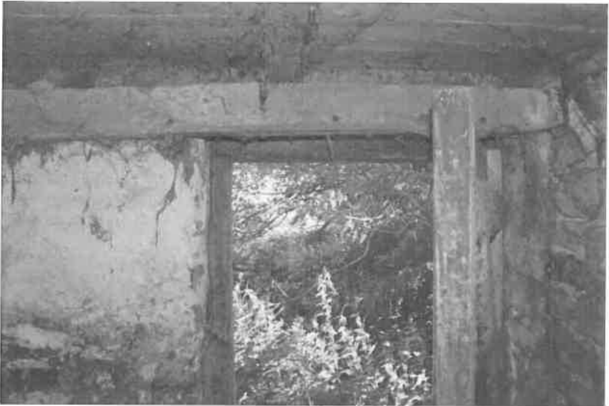
65 The timber beam over the door opening showing notches to the vertical face and the rebate to the stone jamb. The door also opens back against the external elevation.
