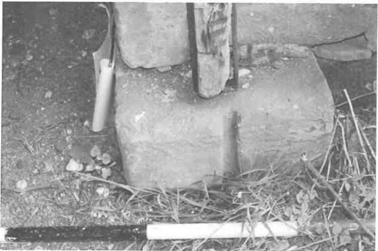
4 The base quoin and slot to the right hand jamb to the cart entrance.
