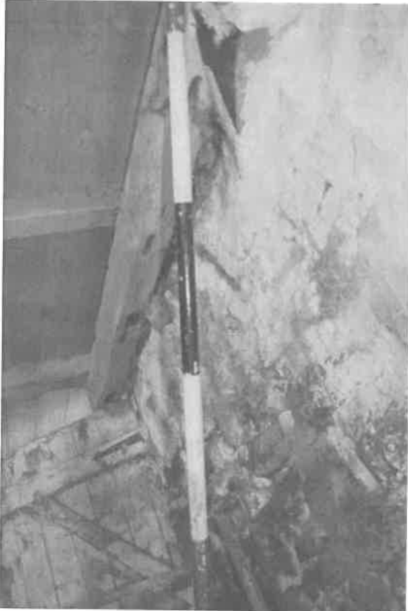
70 The notches to the under-side of the beam to the gable end, with the corbel stone just visible to the top of the image.
