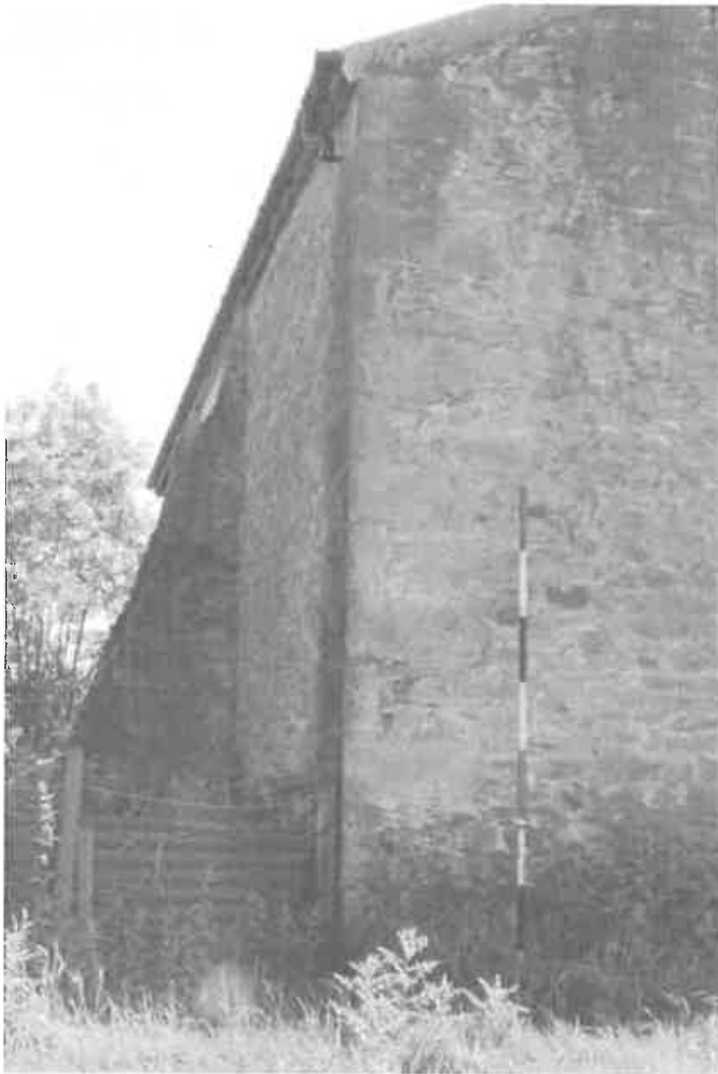
30 The corner of the north west and north east elevations of the barn, showing the quoin detail.
