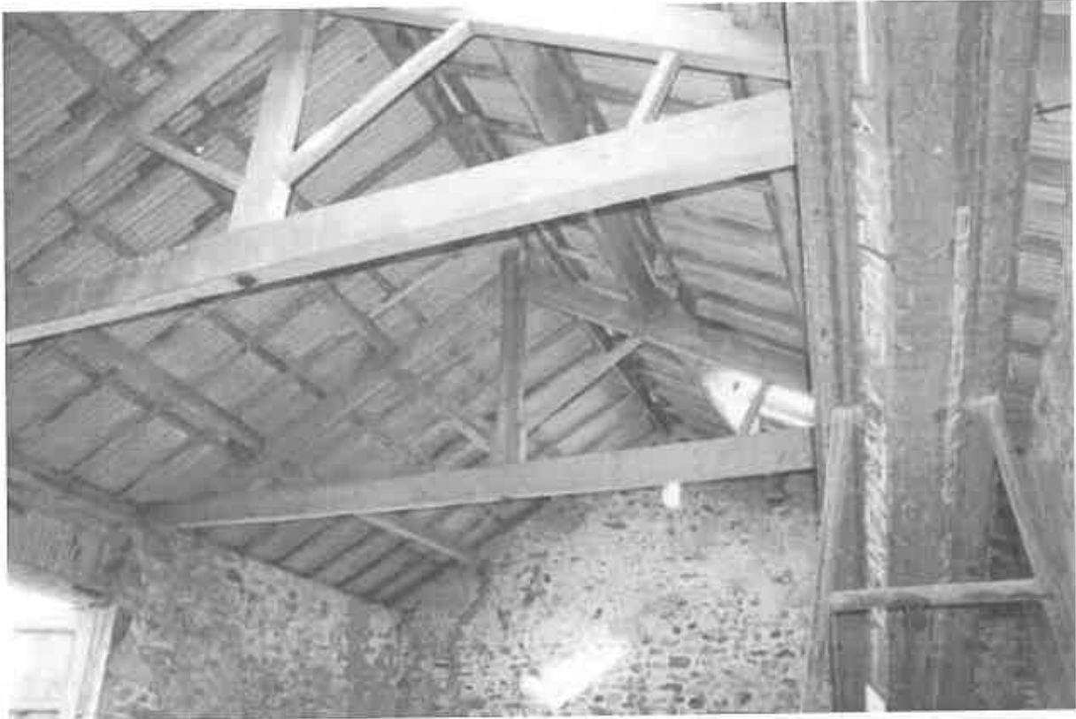
48 The roof structure as viewed towards the south east, showing the tie beam, bracing struts, king joggle post, principal rafters and purlins.
