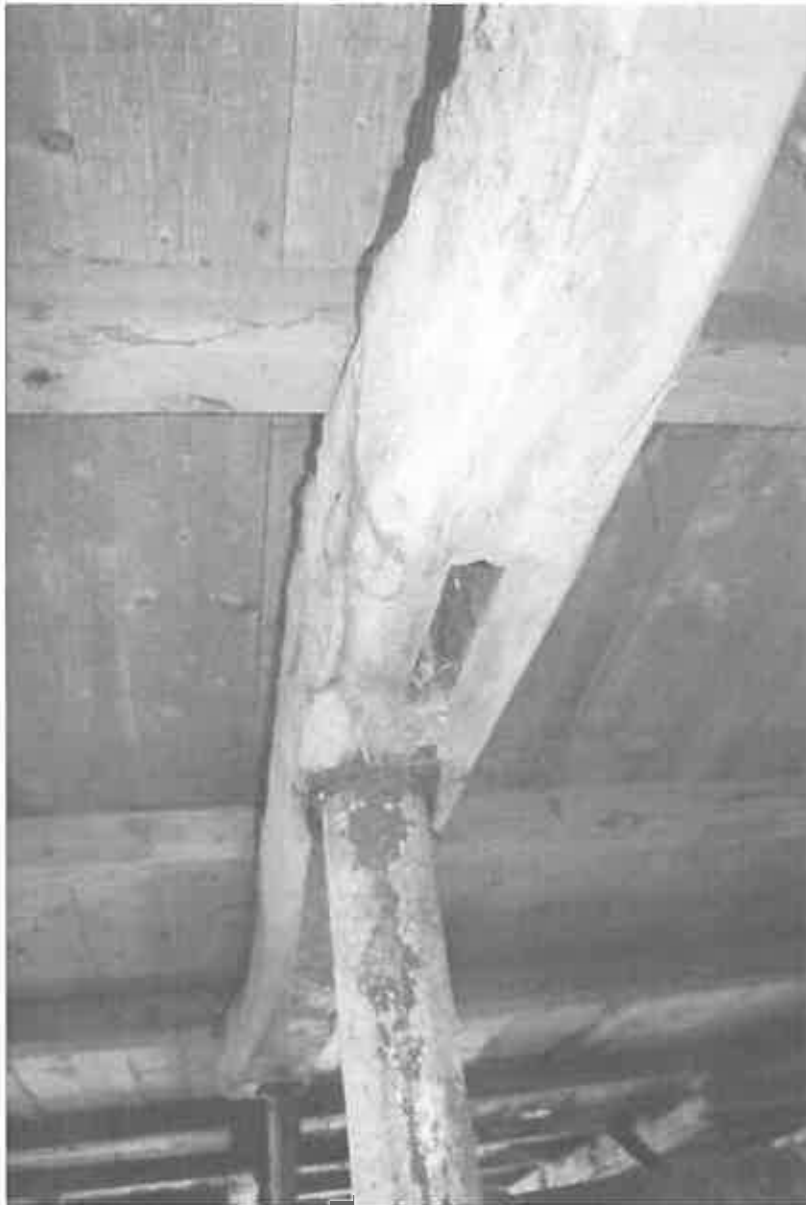
59 A notch to the underside of the floor beams.
