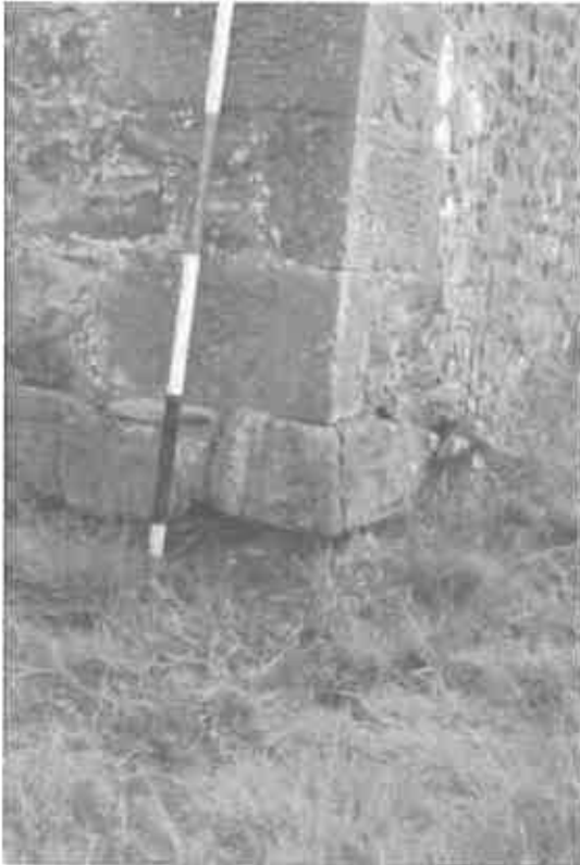
Figure 29 The north west corner – showing the protruding quoin to the base.
