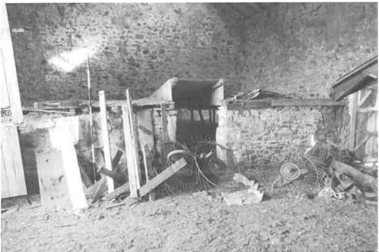
43 The south east gable and the dividing partition with the central doorway through to the lower shippon. The joist ends supporting the timber 'deck' are visible to left hand side..
