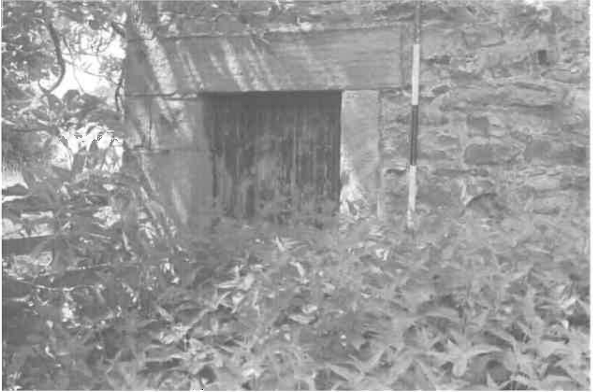
16 The lintel and stone reveals/jambs to the left hand door to the south east gable elevation.
