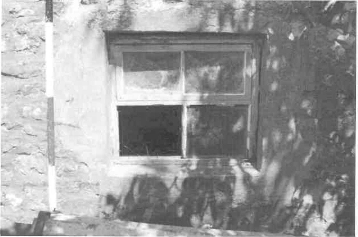
21 The window opening to the south west elevation, showing the two light four pane window. The upper light was top hinged.
