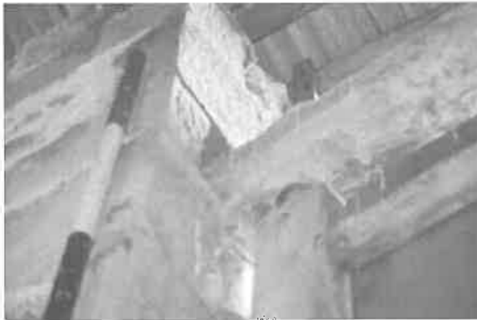
Figure 22 The upper part of the right hand cart bay, with the top of the door set into the cross beam/lintel.
