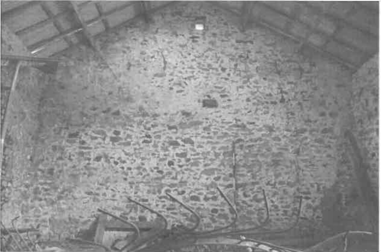
32 The north west internal elevation, with the coursed rubble stonework. The owl hole is also visible towards the ridge.
