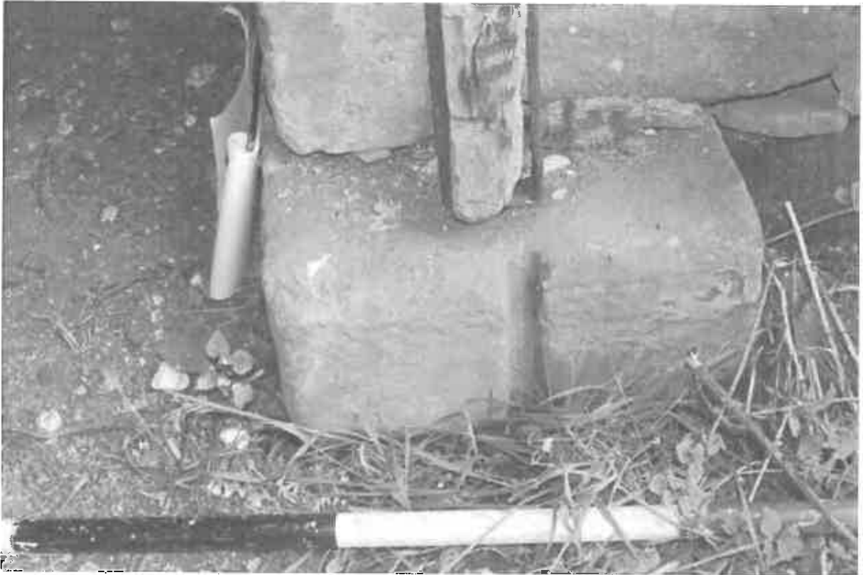
36 The base quoin to the northern side of the cart entrance. The slot or groove for a plank is clearly visible.
