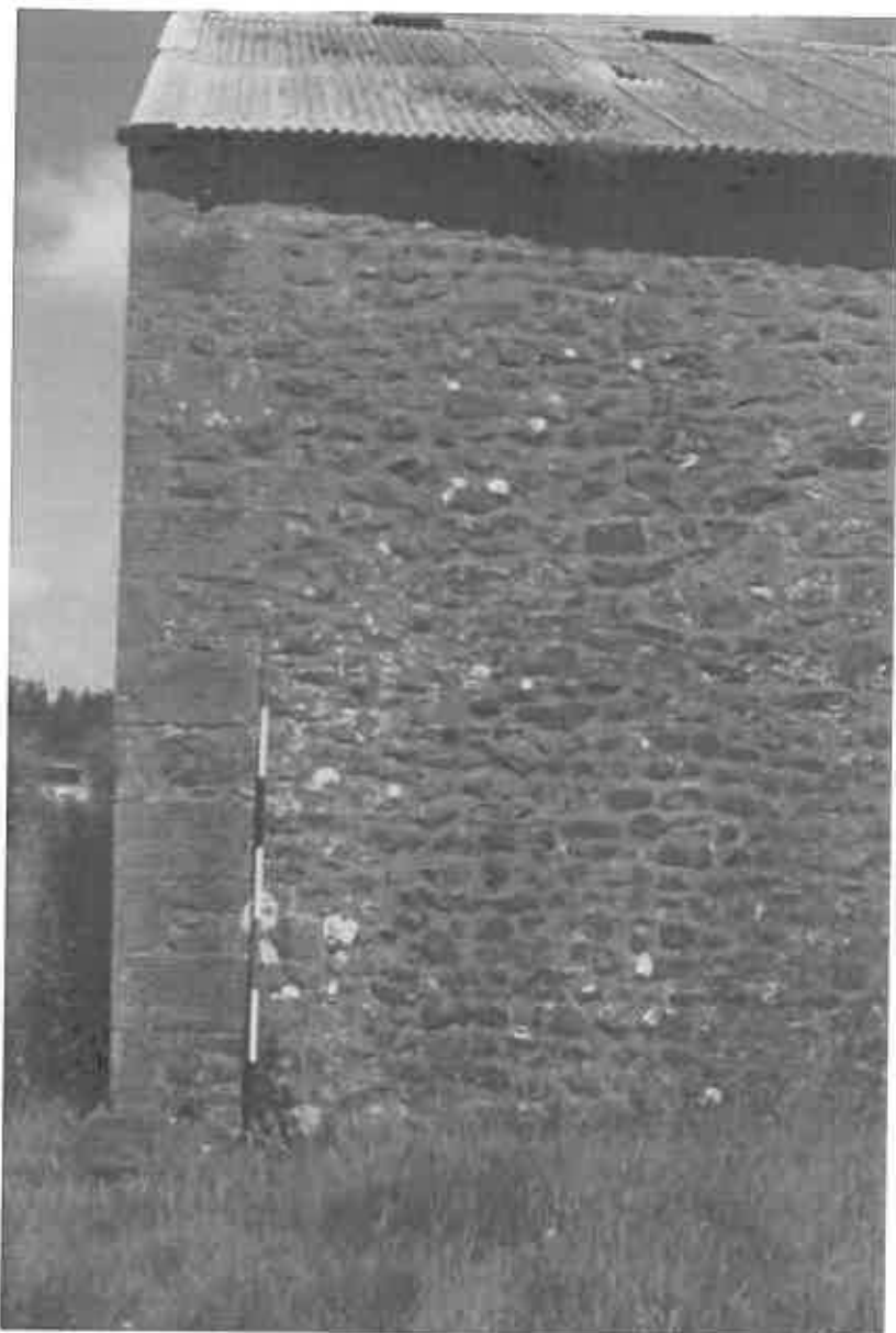
25 The north west corner, showing the quoin detail and the protruding base quoin.
