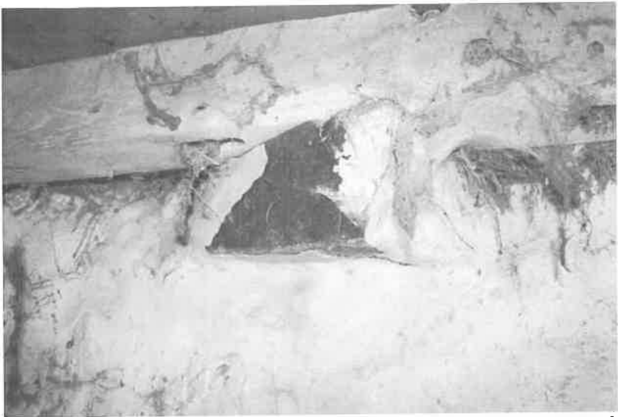
68 The stone to between the central door and the door opening to the south west corner of the gable. This may have been a corbel, but it stands in isolation.
