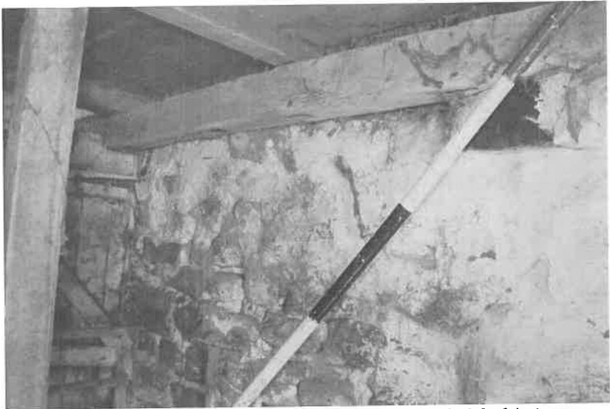
71 The timber beam to the gable end, with the central doorway to the left of the image. The notches are just visible to the underside of the timber.
