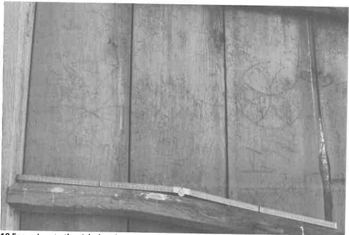
10 Engravings to the right hand cart entrance door
