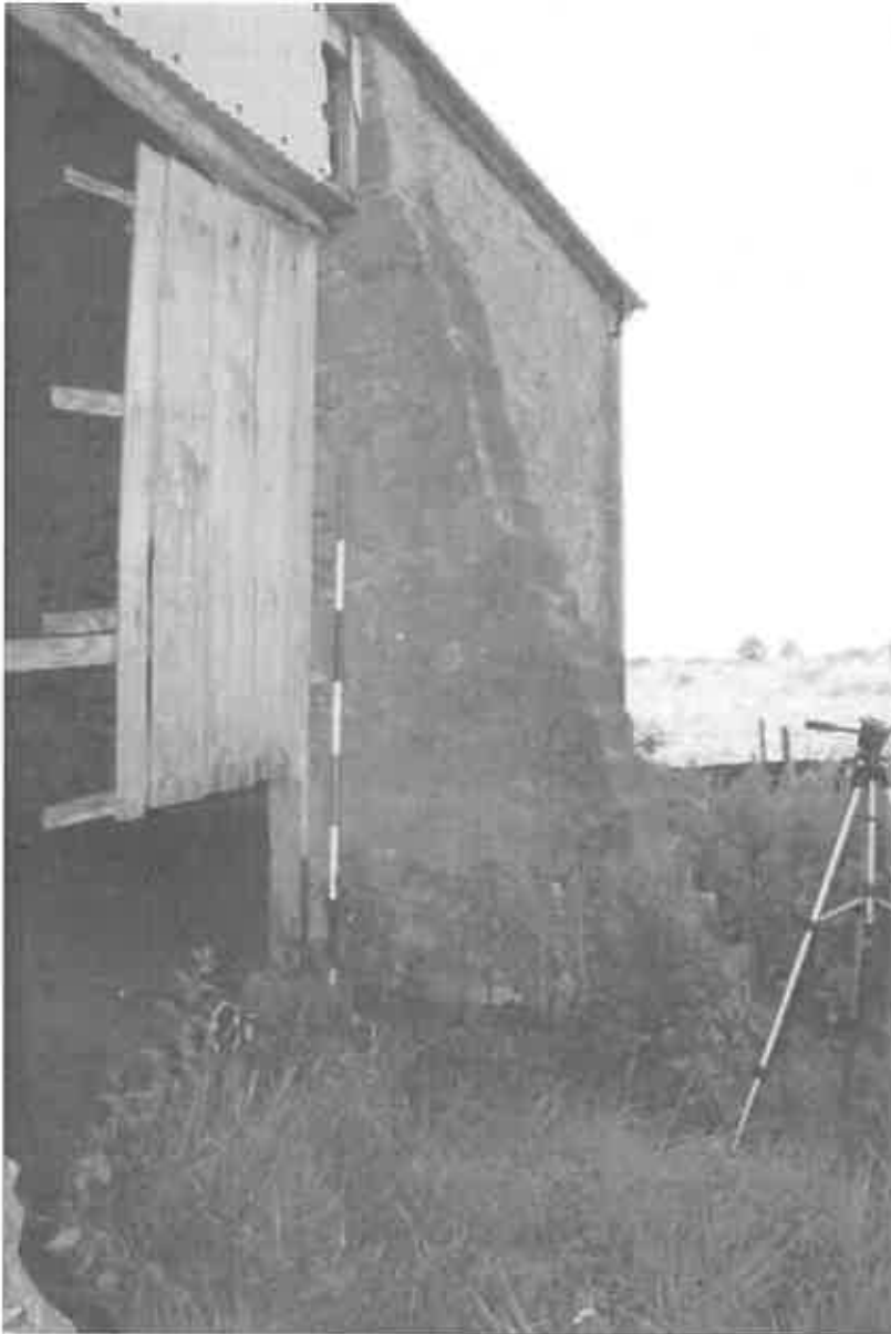
7 The right hand buttress, with some of the quoin detail to the entrance jamb visible in the buttress stonework.
