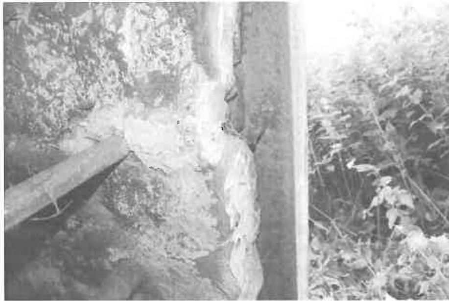
Figure 47 The rebate to the door opening to the right at the gable end.
