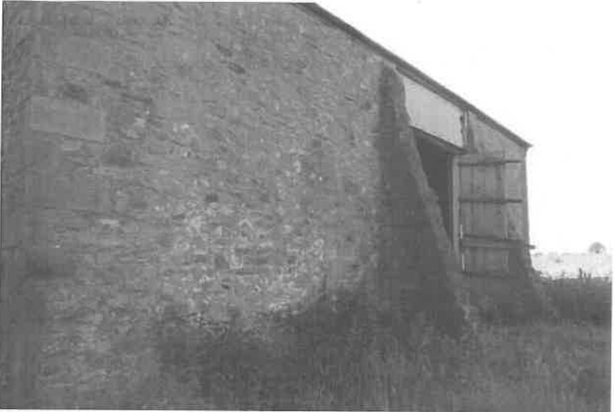
3 The buttresses as viewed from the south west, with quoin detail to the south west corner also seen.
