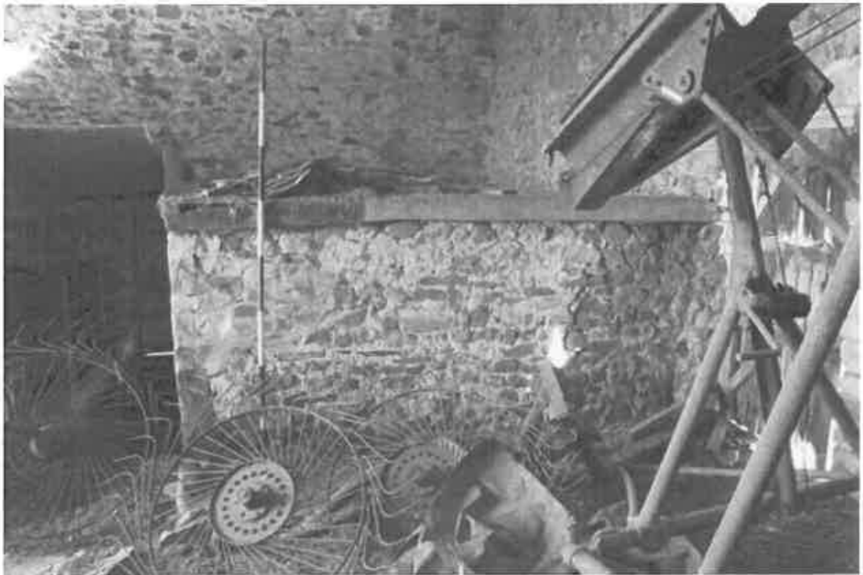
45 A view of the internal partition, formed mainly in coursed rubble stone, with some brick infill.
