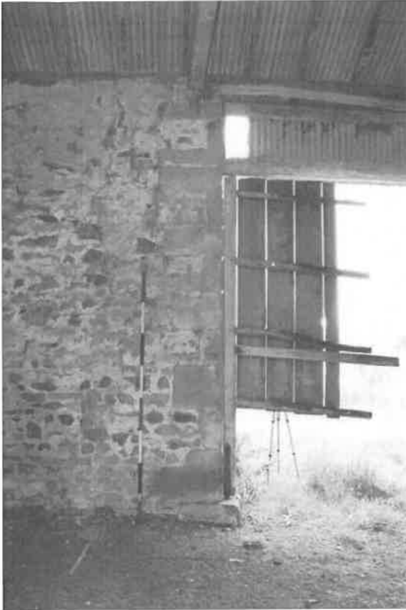
35 The internal jamb of the cart entrance, showing the quoin detail and the protruding base quoin.
