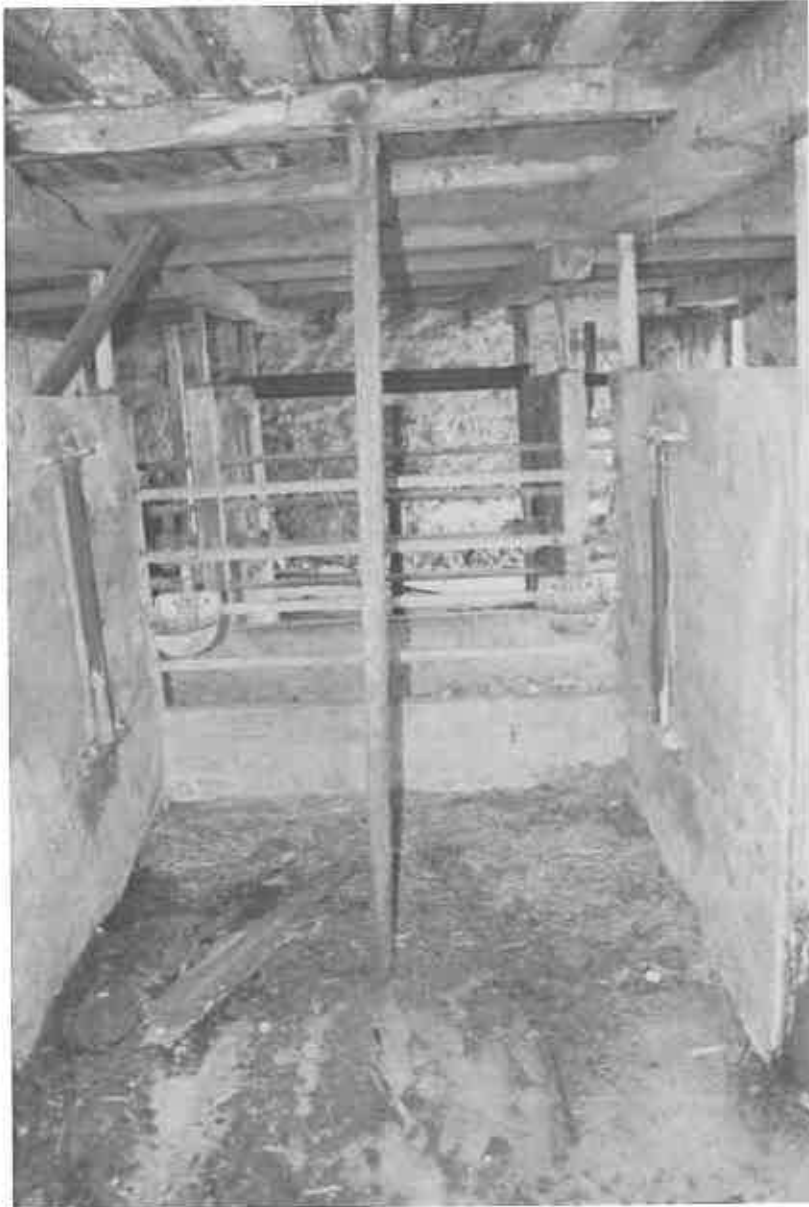
73 A view across the central stall to the south west side of the shippon, showing the floor joists and additional beam and the extra supporting pole added for the upper 'deck'
