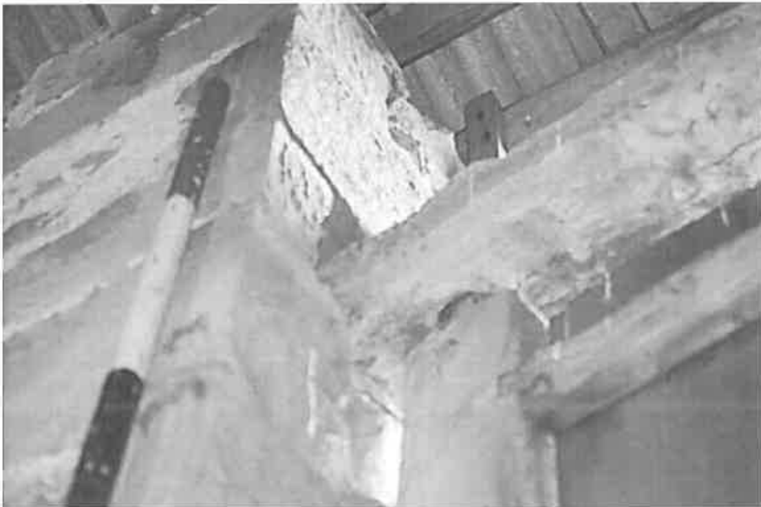
40 The upper hinge to the northern cart door, formed by a recess into the cross beam.
