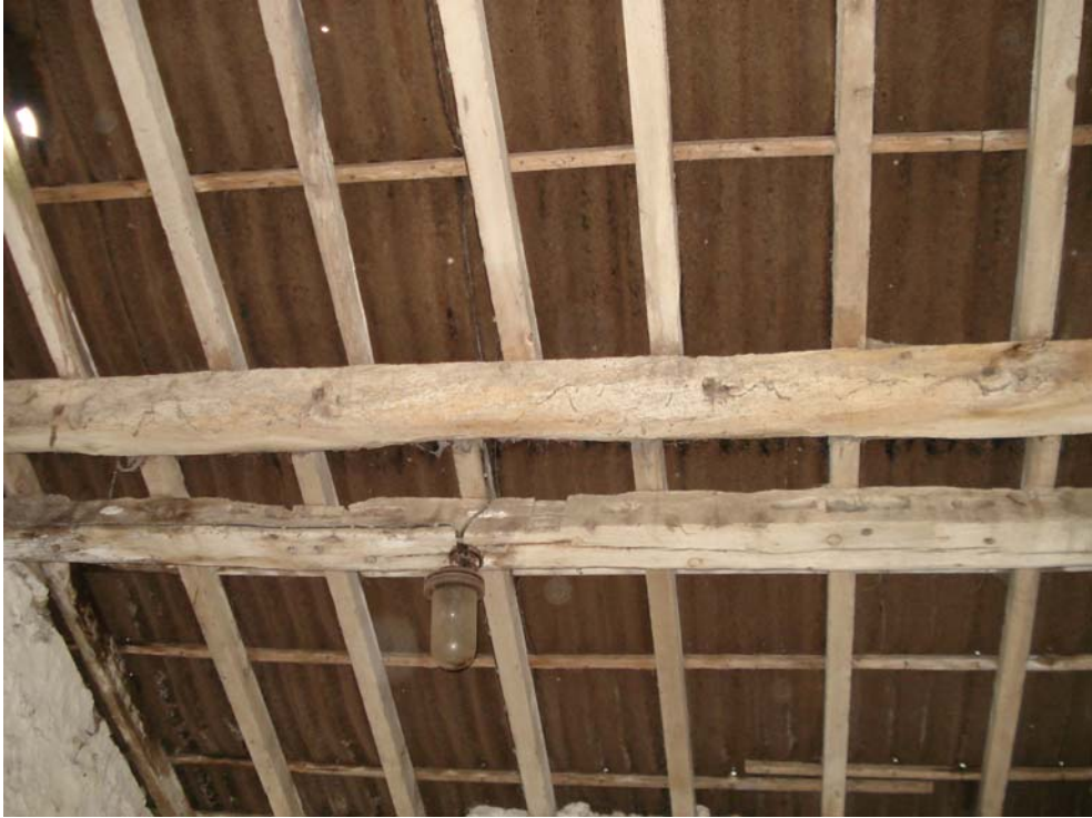
Plate 29 – Purlin section depletion (Shippon)
