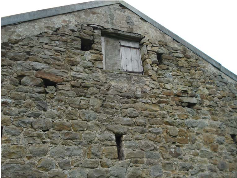
Plate 3 – Weathered mortar to North gable apex
