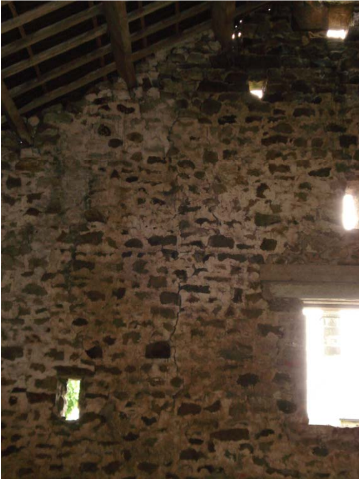
Plate 19 – Vertical cracking to inner leaf (South Gable)
