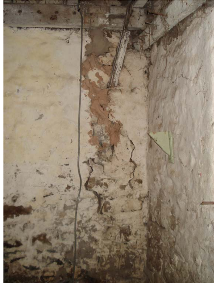
Plate 36 – Vertical crack, damp penetration to applied Shippon wall finishes
