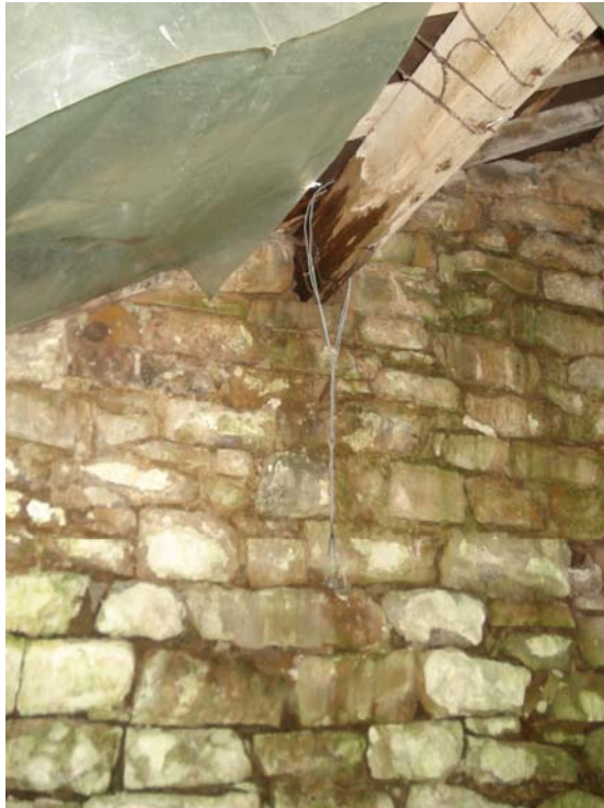
Plate 31 – Damp penetration to purlin bearing at North gable (Shippon)
