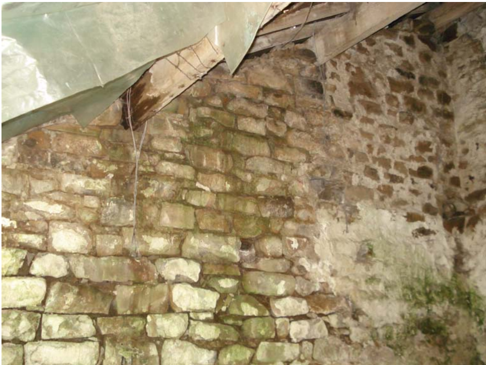
Plate 30 – Damp penetration to purlin bearing and North gable (Shippon)
