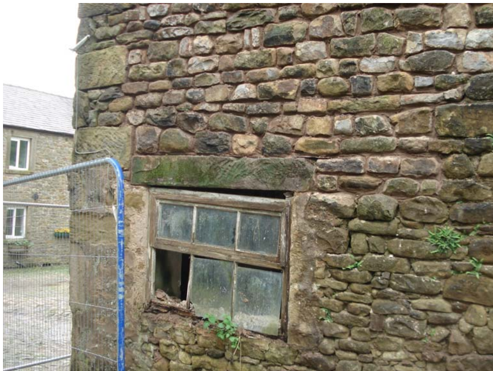
Plate 8 – Lintel bearing movement
