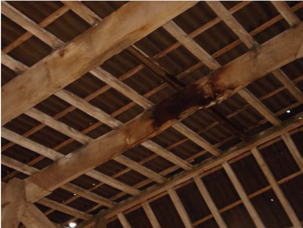
Plate 17 – Damp and rot to purlin
