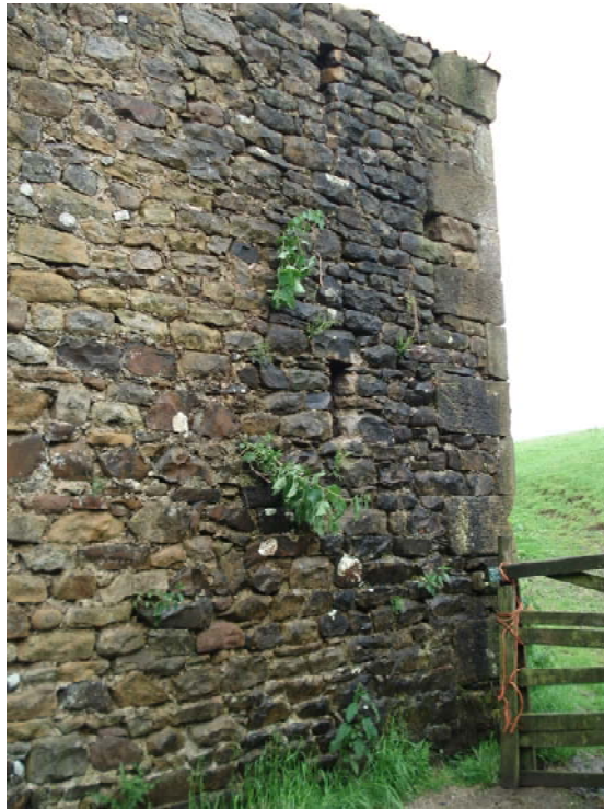
Plate 7 – Water staining and vegetation growth
