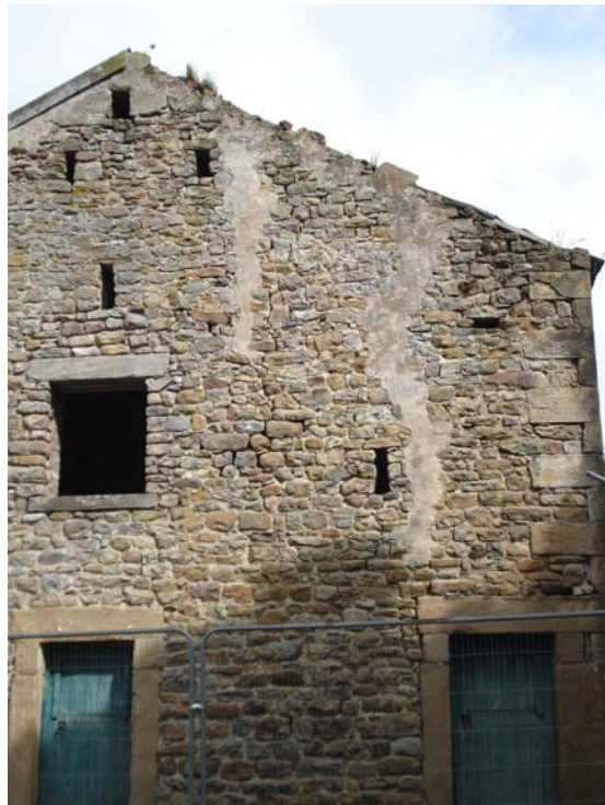
Plate 10 – 'Re-pointed' masonry cracking
