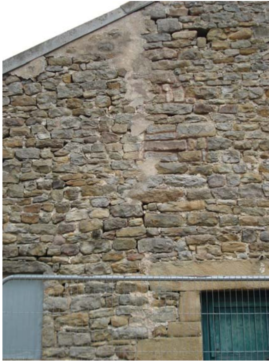
Plate 11 – ‘Re-pointed’ masonry cracking (‘Shippon’)
