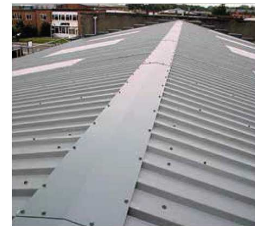
Profiled roof cladding with translucent rooflights
