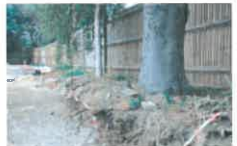
Potential loss of existing tree due to poor construction techniques.
