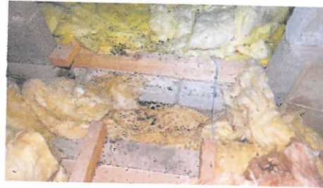
Figure 9: fresh bat droppings void 'A'
