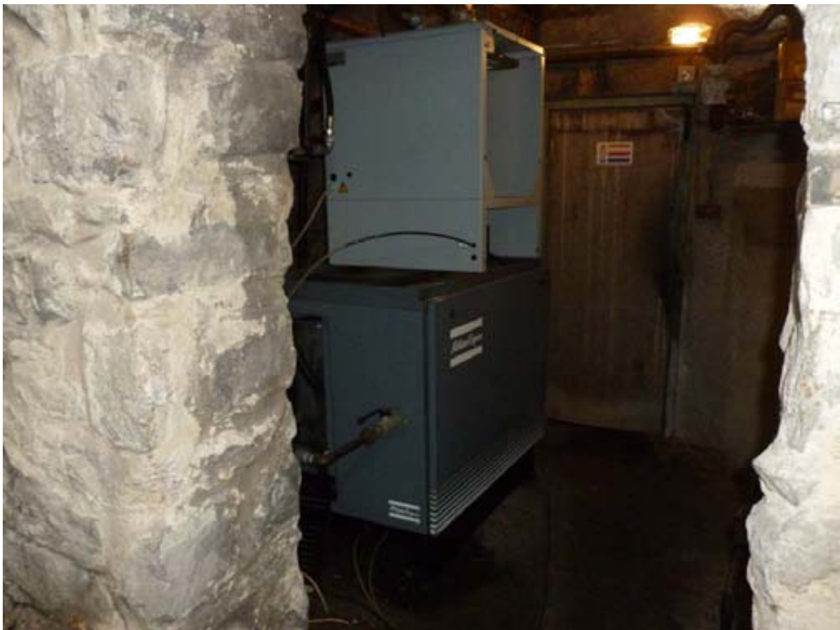
Photo 14 – Gas fired boiler within W end of basement, looking NE.
