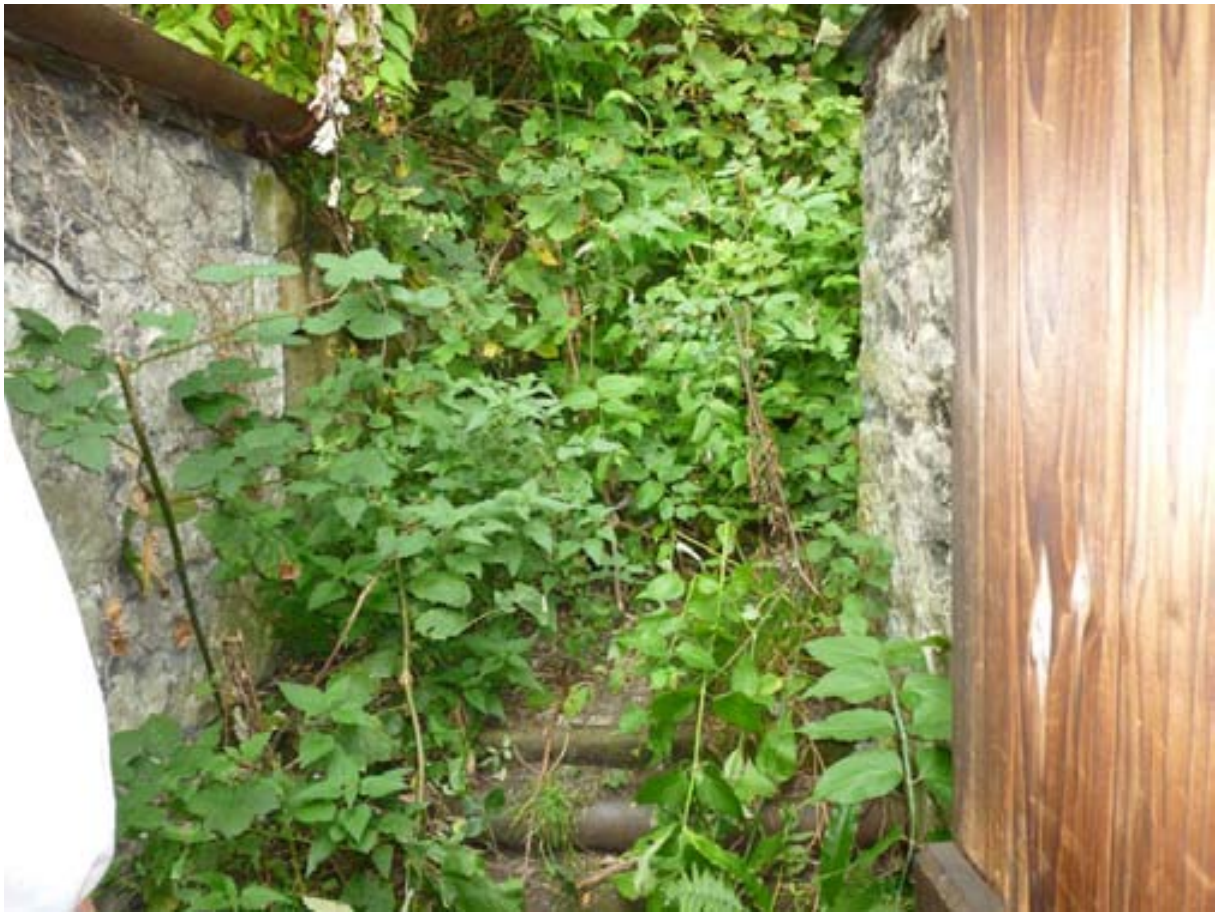
Photo 15 – Overgrown yard on slope, to W of S building, looking N.
