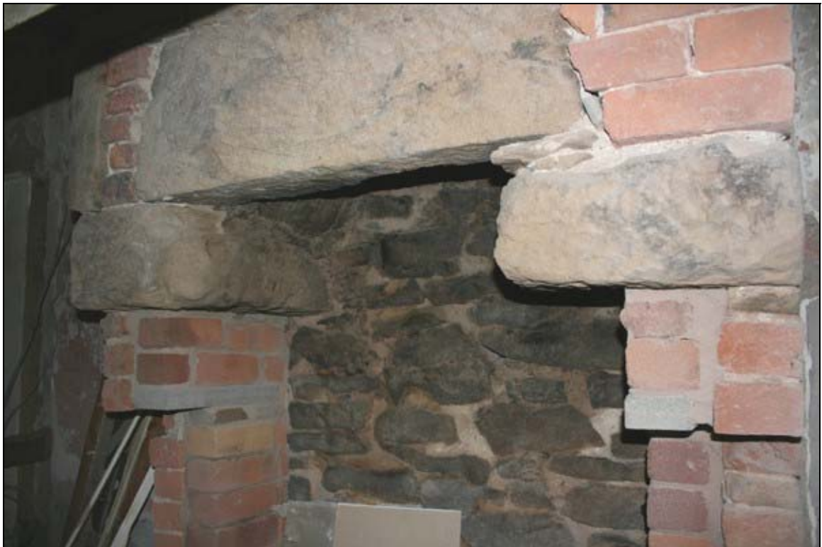
14. Fireplace beneath firehood has experienced modern alteration
