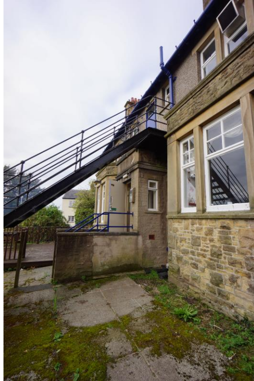
Figure 1 Unightly fire escape and modern porch concealing the original stone surrounds to the former rear entrance
