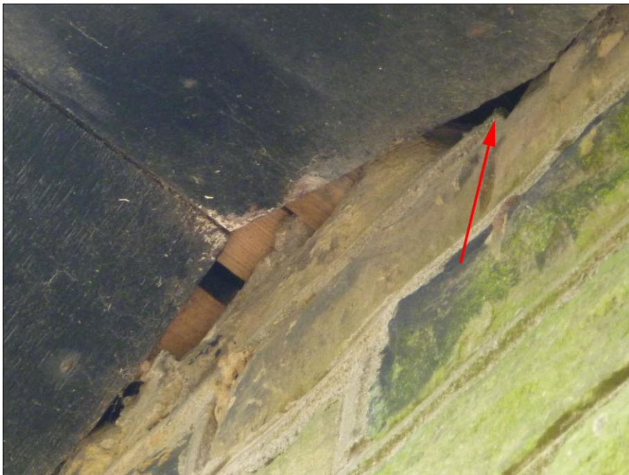
Plate 3: Gaps where bats could gain access were observed on the garage end gable under the soffit boards
