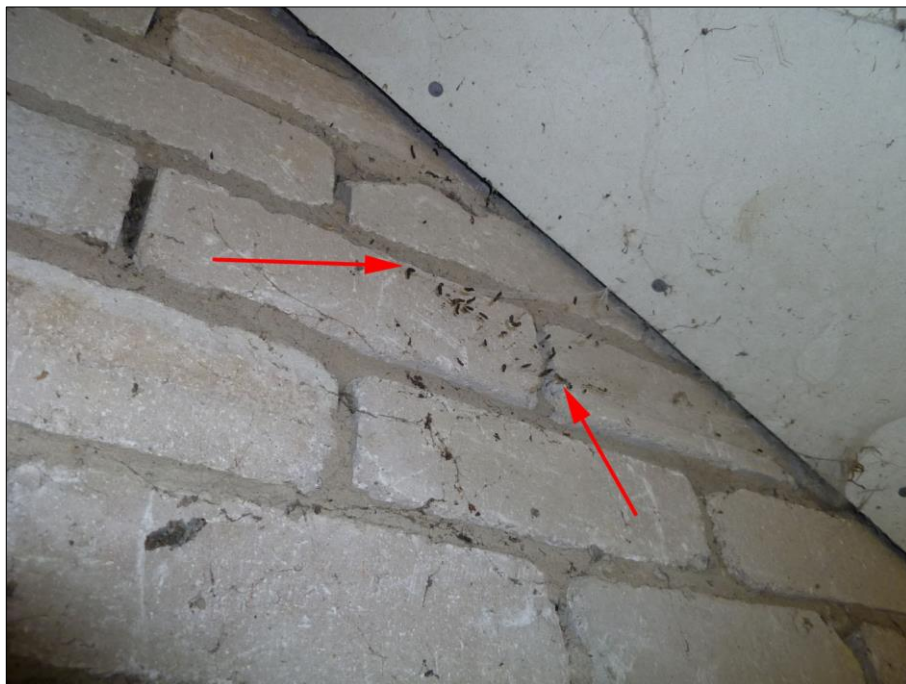
Plate 14: Bat dropping discovered on interior wall caught within cobwebs indicating bat presence
