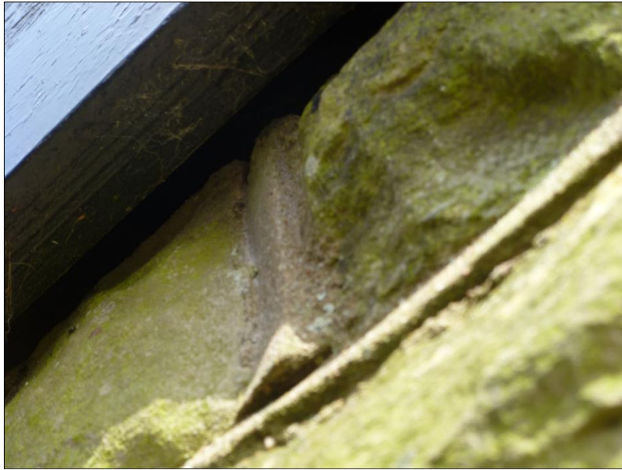
Plate 6: Gaps between the fascia board and wall could allow bat access
