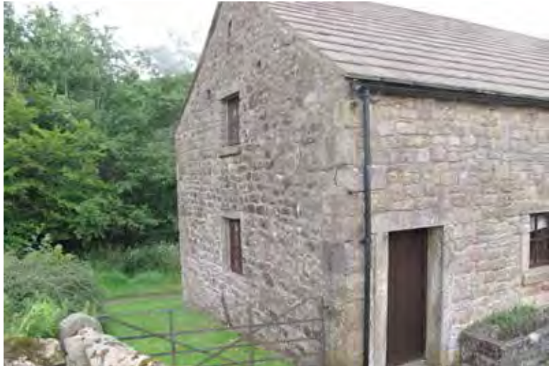
Photograph 34. The windows in the west gable wall appear to have been inserted as part of the conversion to a camping barn.
