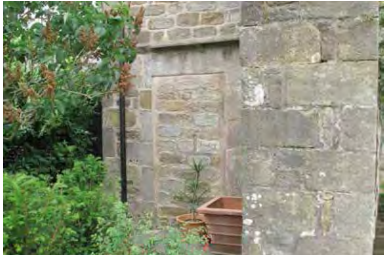
Photograph 10. The blocked original doorway at the left-hand end of the facade. The quoins at this corner do not support the suggestion that the building originally extended further to the west.
