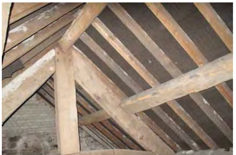
Photograph 28. The purlins show evidence of re-use. The softwood rafters date from the re-roofing circa 1980.
