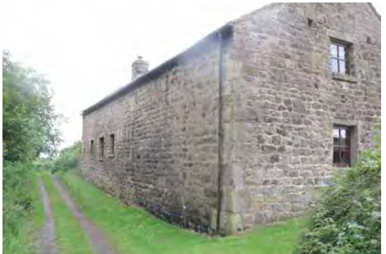
Photograph 35. The north side of the former shippon. Some lime mortar pointing and some of the original breather holes remain.
