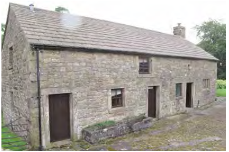
Photograph 33. The south side of the former shippon. The stone surrounds to the doorways and some of the windows have tooling typical of the early / mid 19th century.
