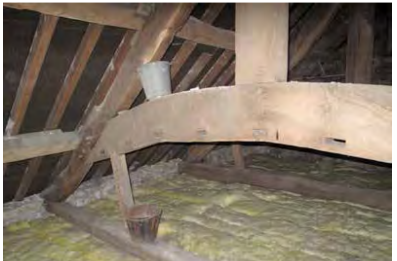
Photograph 27. The roof trusses are of an unusual design with mortices in the sides of the curved collars.
