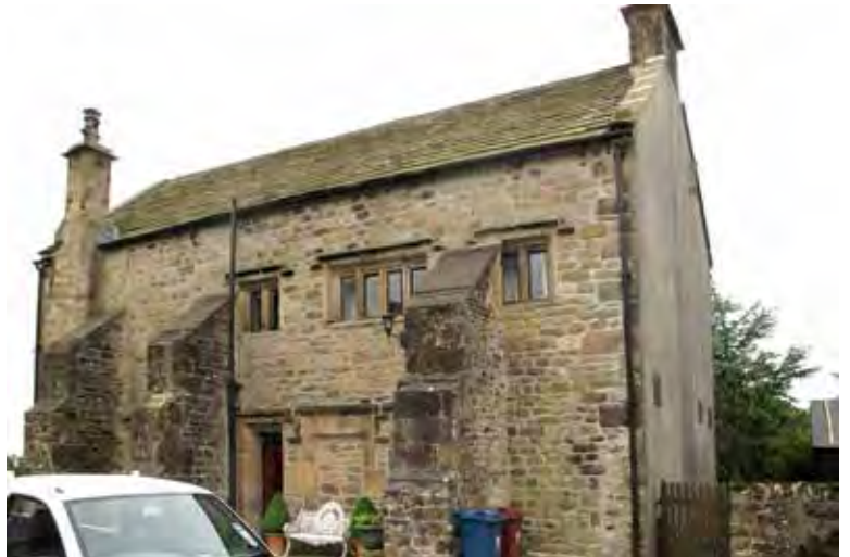
Photograph 14. The north side of the house. The west gable wall was underpinned and rendered with cement about 35 years ago.
