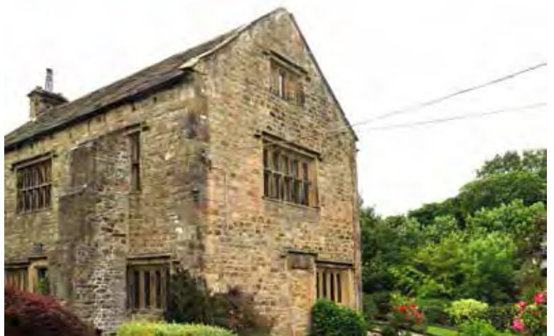
Photograph 12. The east gable. The blocked ground-floor doorway is particularly narrow and has a blank wall to its left. The attic was lit by a 3-light window.
