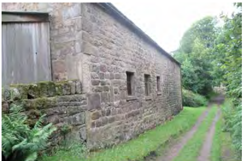
Photograph 36. The north side of the former shippon. The window openings appear to have been inserted when this end of the building was converted into a holiday cottage.
