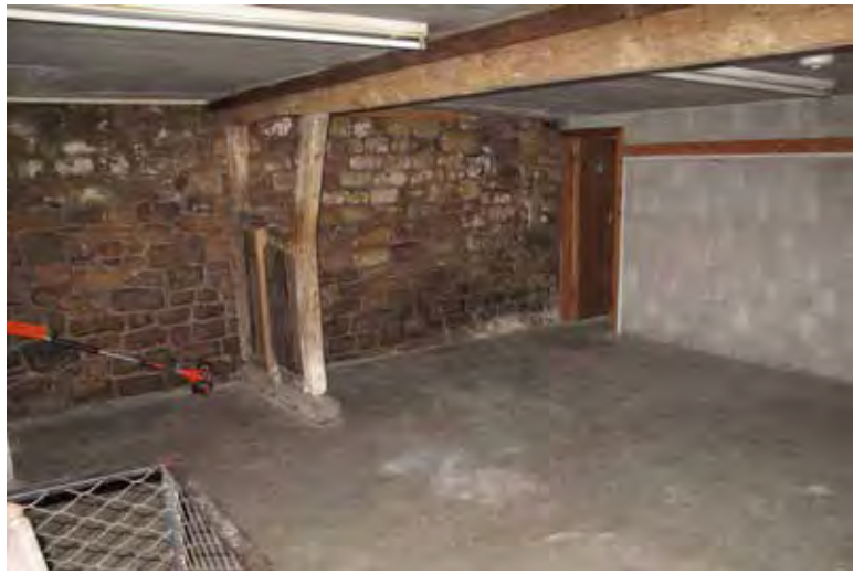
Photograph 37. The ground floor of the camping barn. A boskin has been retained to show its former use as a shippon.
