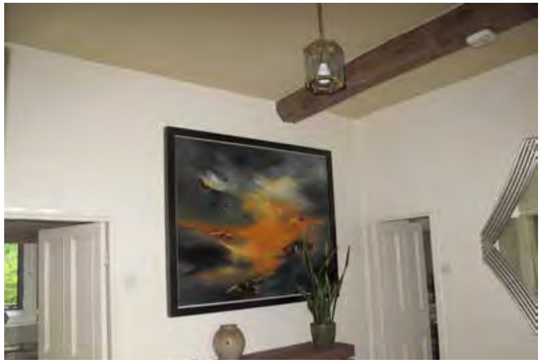
Photograph 25. The first floor landing. The deeply-chamfered ceiling beam is original but there is a separate tie beam to the truss in the loft above.
