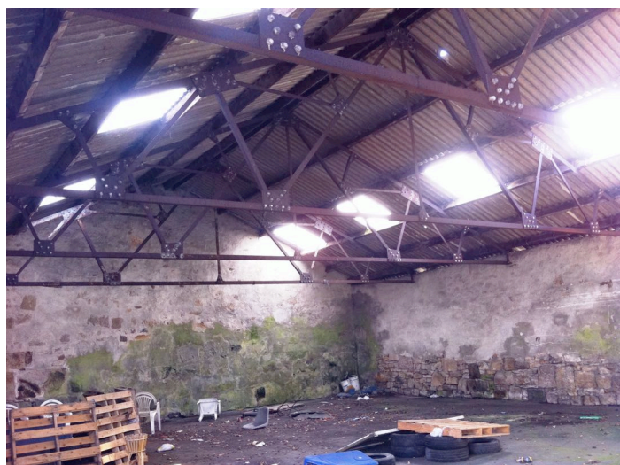
Photo 6. Internal view of the section of building proposed for removal, looking towards the gable end
