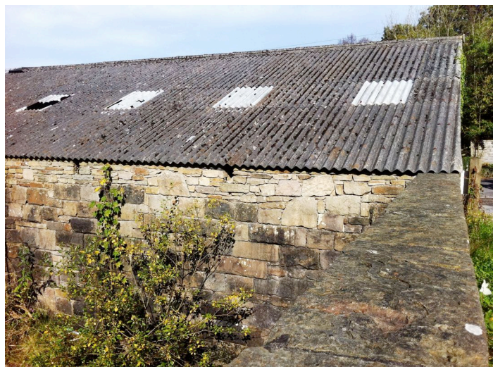
Photo 2. Close up of the roof of the section of building proposed for removal
