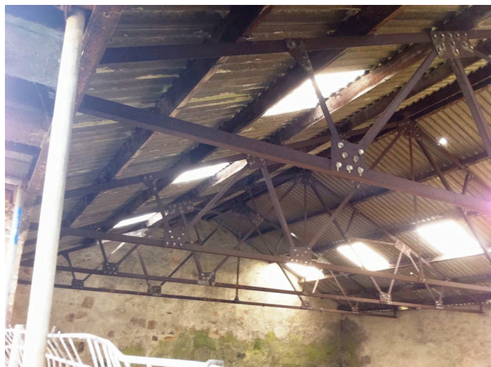
Photo 9. Internal view of the section of building proposed for removal, clearly showing the corrugated roof sheets supported on steel framework
