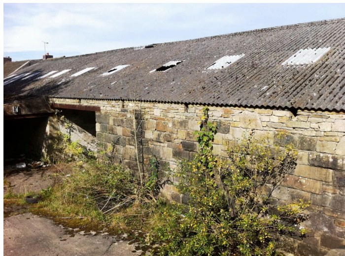
Photo 3. Detailed view of the rear wall of the section of building proposed for removal
