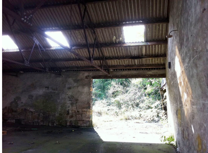
Photo 7. Internal view of the section of building proposed for removal looking towards the opening to the rear
