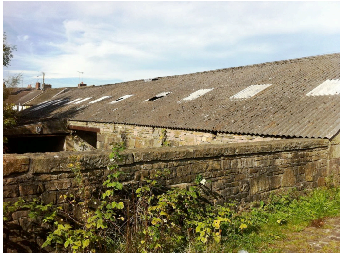
Photo 1. The roof and rear elevation of the section of building proposed for removal
