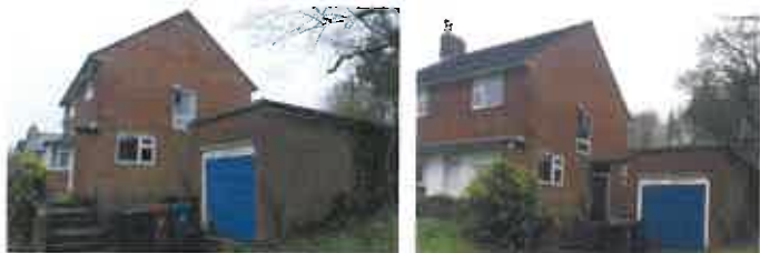
Side north east elevation of house and single storey section to be demolished
