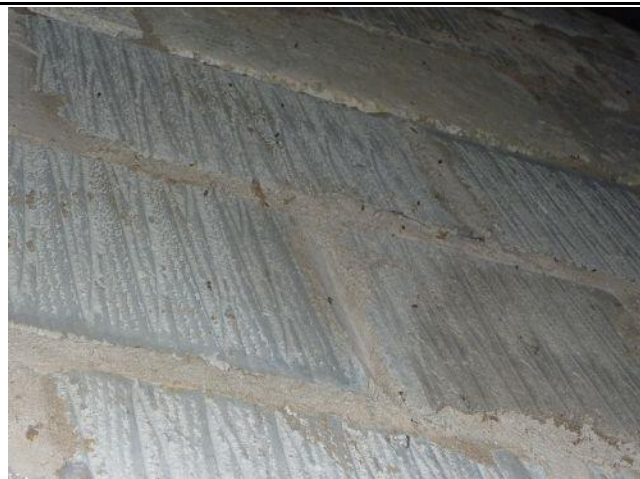
Photo 13: Building 1, approximately 30 scattered bat droppings (all old) on internal wall, under western gable end (Roost 1.1)
