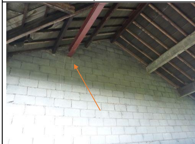
Photo 20: Building 1, barn owl faecal splashing at central open sided section
