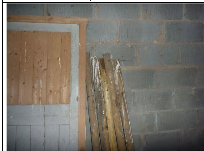
Photo 22: Building 1, faecal splashing at internal wall of eastern gable end, eastern end of the building.
